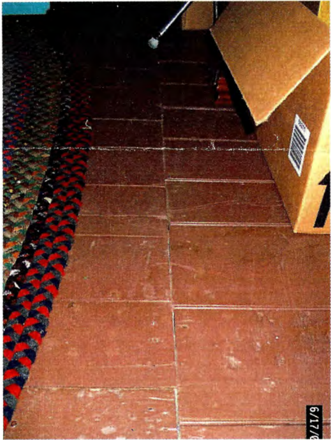
Upper level wood floor showing where planks were added, possibly covering an earlier stairs.
