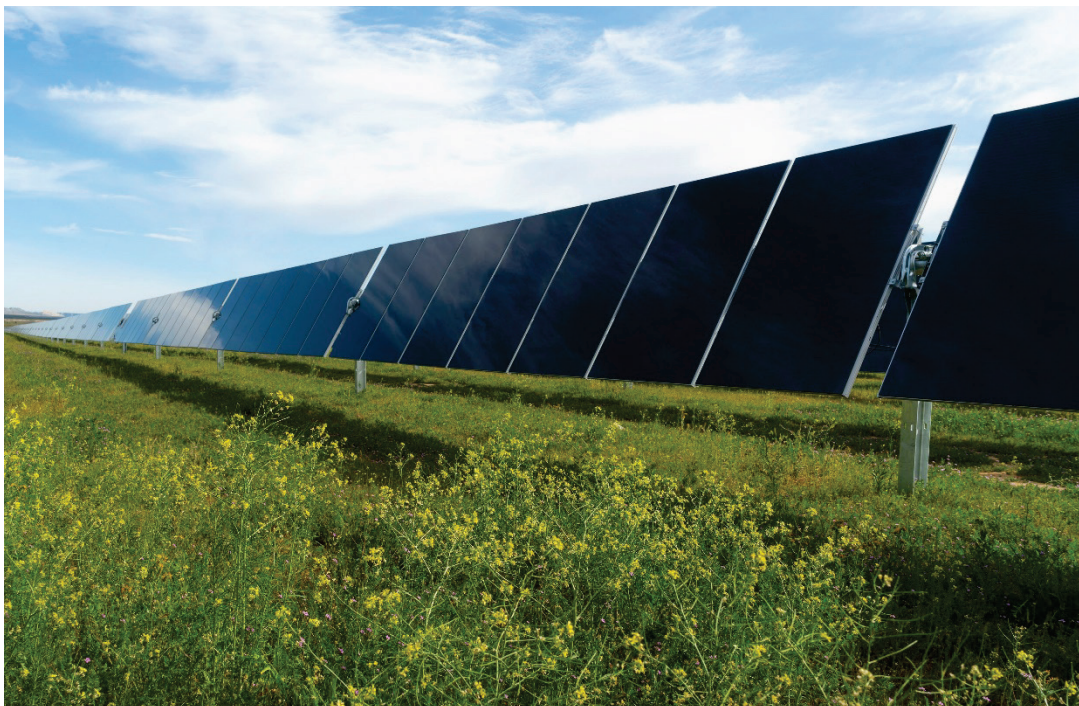
Photo 3-5. Single-axis, tracking photovoltaic system with panels near maximum tilt as viewed from the east or west
