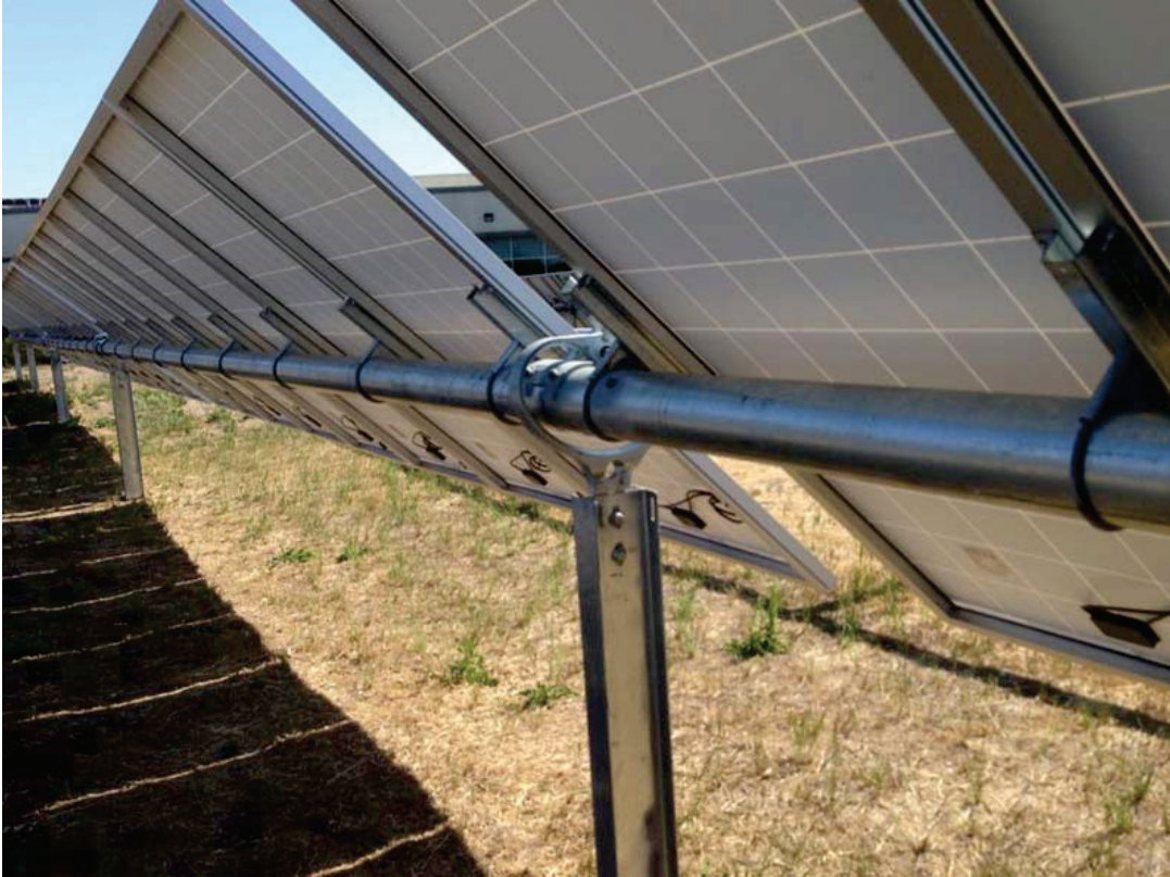
Photo 3-6. The backside of the solar panels in early morning or late afternoon configuration
