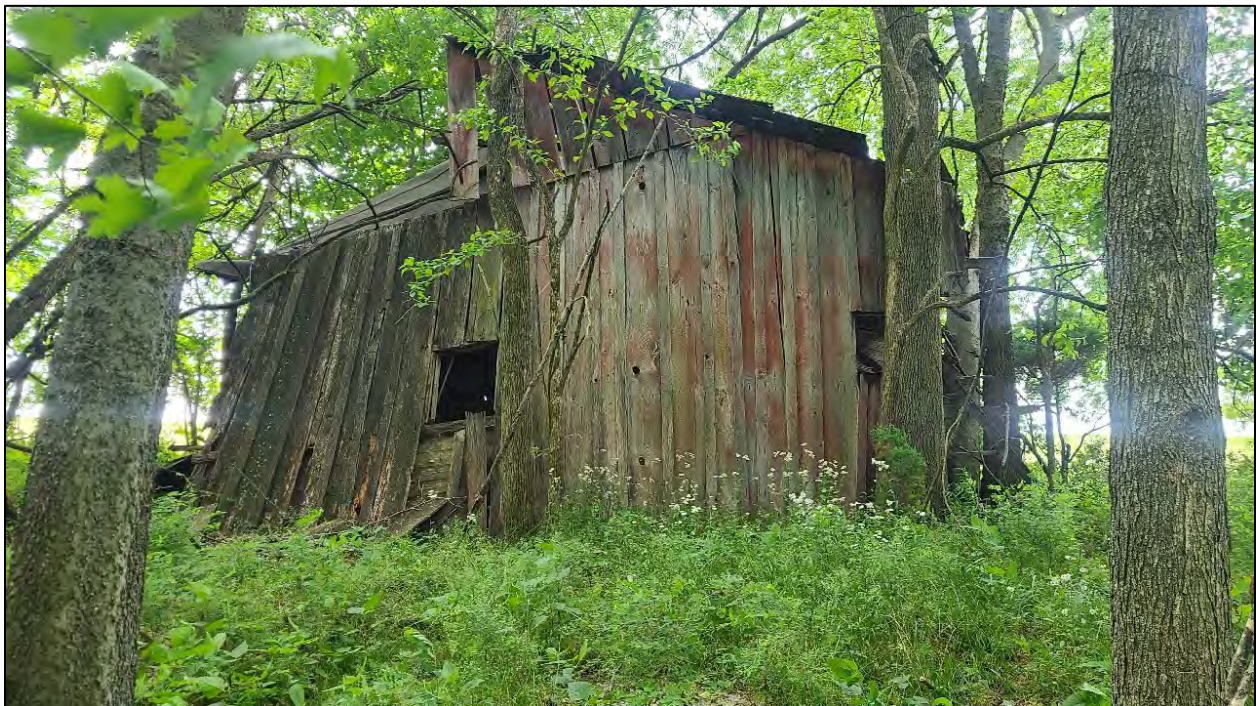
Photograph 2 – Dilapidated barn on Project Area parcel 055-00-00-006-00, view to the east.
