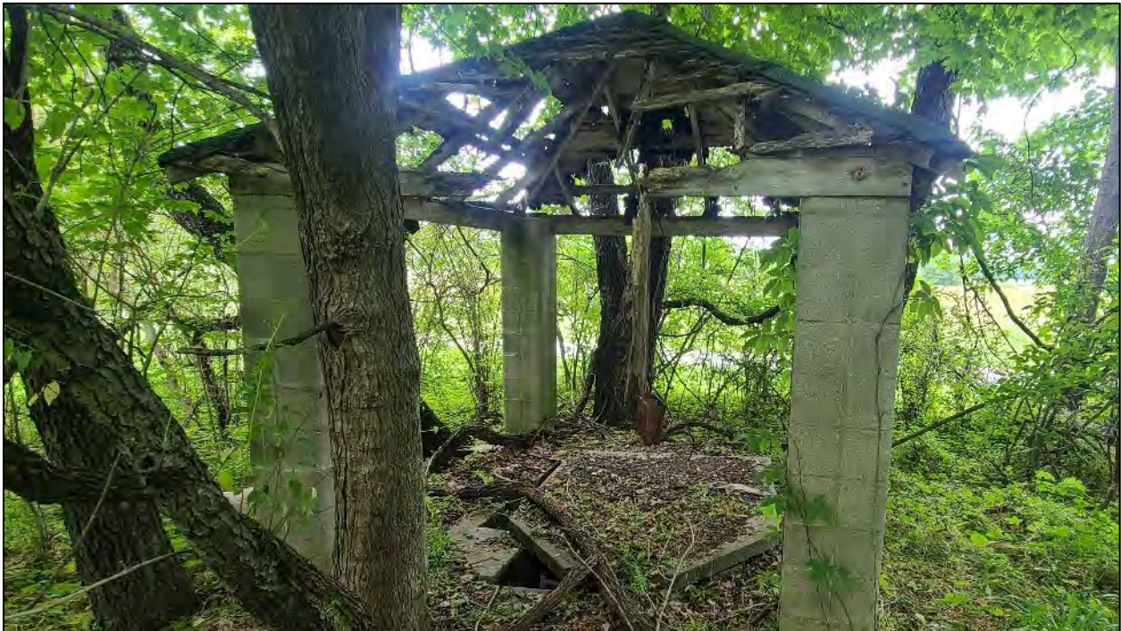
Photograph 14 – Homestead pump house on Project Area parcel 055-00-00-016-00 and J Montgomery Road, view to the west.
