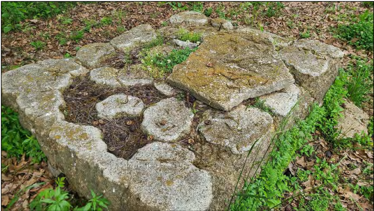
Photograph 28 – Concrete pad with bolt anchors on Project Area parcel 041-00-00-005-00, view to the southwest.
