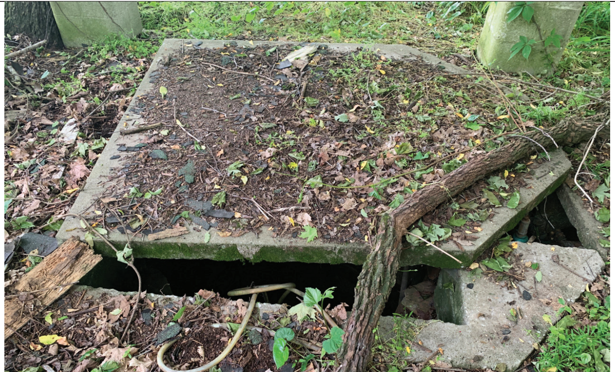
Photograph 42 – Old home site concrete pump site, forest stand 16, gray bat roosting habitat, facing northeast
