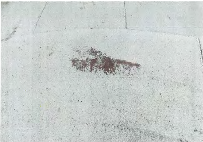
Photo shows a closer view of delamination on the west portion of the roof.
