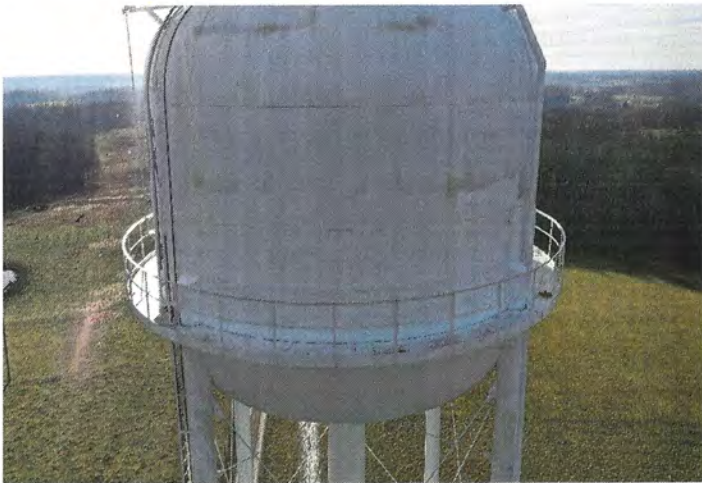
Photo shows an overall view of the north shell. Areas of blotchy corrosion are visible. The coating system has reached the end of its life cycle.
