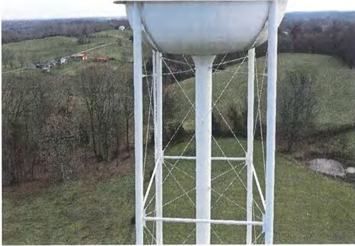
Photo shows the west side upper panel. Mildew is visible on the lower knuckle panels.
