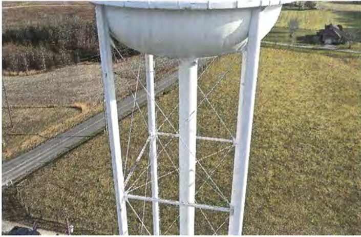
Photo shows the west upper panel members. The windage rods and struts are properly aligned.
