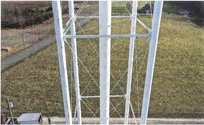
Photo shows the middle west side panel. The white finish coat shows signs of erosion.
