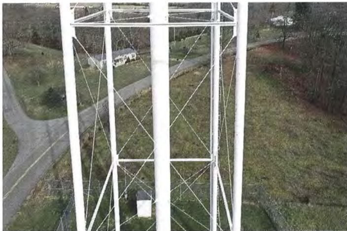
Photo shows the middle south side panel members. All rods appear to be properly adjusted. All connections appear to be sound.
