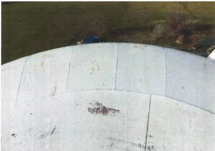
Photo shows the west portion of the roof. General corrosion and delamination to the red primer was noted.
