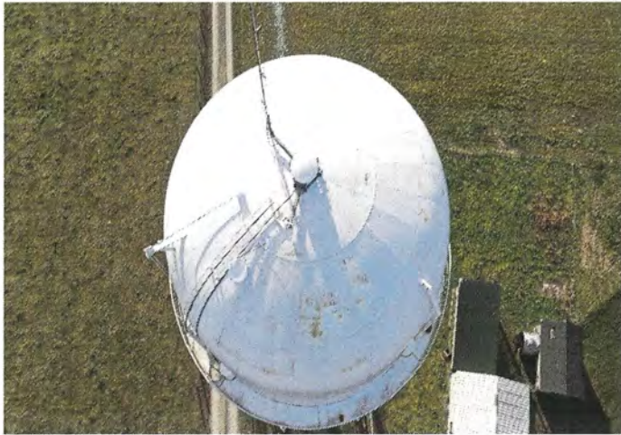
Photo shows an overall view of the roof. The white finish coat has lost its gloss but continues to protect the steel substrate.
