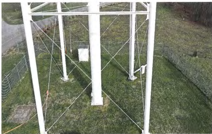
Photo shows the lower portion of the legs on the south side. The white urethane finish coat is very close to the end of its life cycle.
