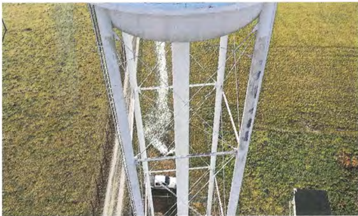
Photo shows the north portion of the upper legs. The coating has eroded on the upper panel leg sections.
