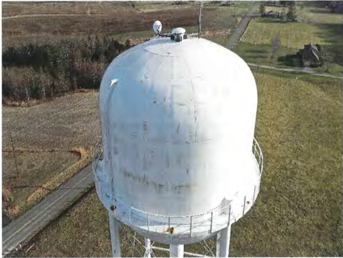
Photo shows an overall view of the west shell. General corrosion was noted along the upper knuckle.
