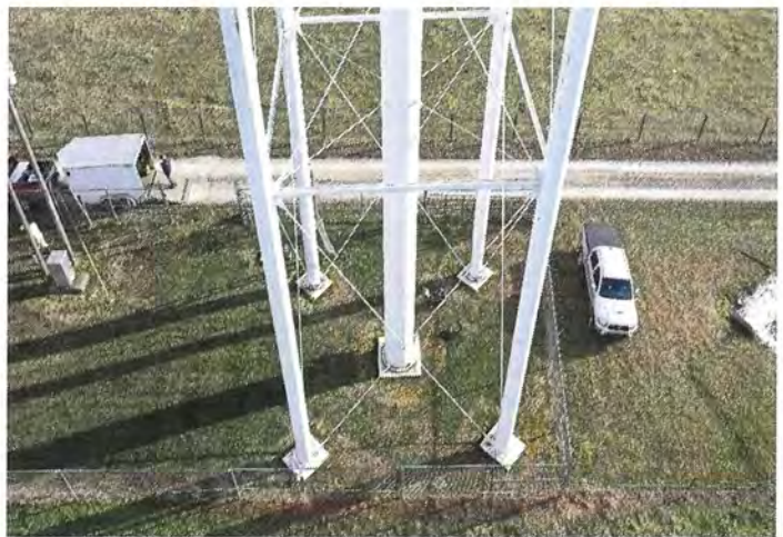
Photo shows the lower west side panel. The tank has three panels and two struts.
