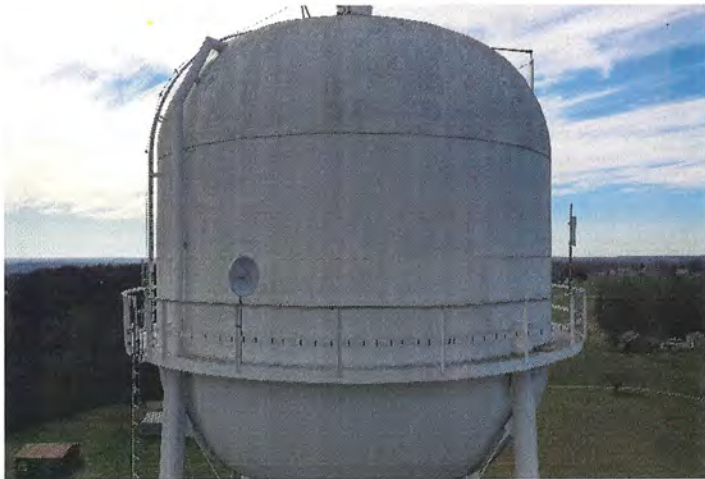
Photo shows the north portion of the shell. The finish coat shows signs of erosion along the upper knuckle.
