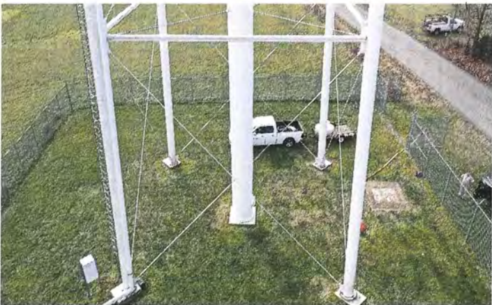
Photo shows the lower portion of the legs on the north side. The white finish coat has lost all of its gloss.
