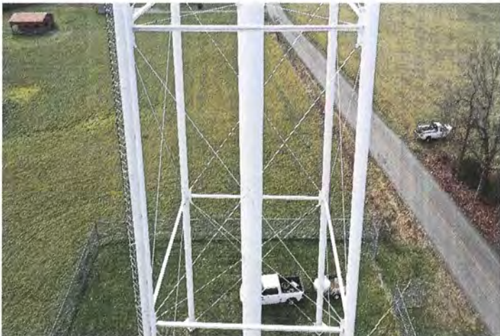
Photo shows the middle north side panel. The pinned rods and strut connections appear to be structurally sound.
