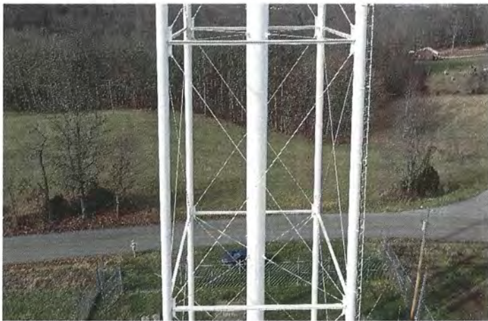
Photo shows the center panel members on the east side. All windage rods appear to be properly adjusted.
