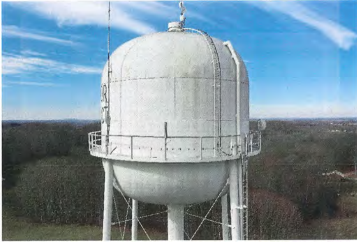
Photo shows the east portion of the shell. The coating has lost its gloss but continues to protect the steel substrate.
