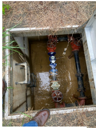
Hickory Road Meter
