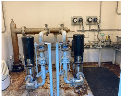
KY 437 Pump Station
