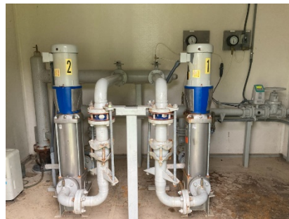
KY 205 Pump Station
