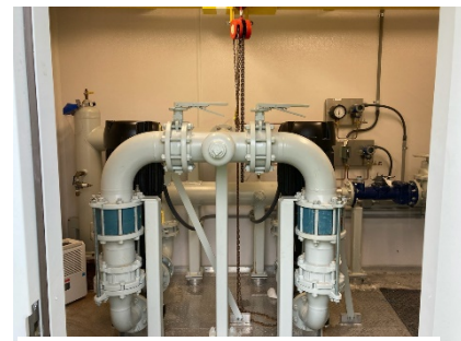
Spaws Creek Pump Station
