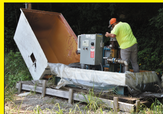
An Alliance Water Resources employee worked on the pump that supplies water to Meathouse and Big Branch Road customers on Route 1439. (Citizen photo by Rachel Dove)
