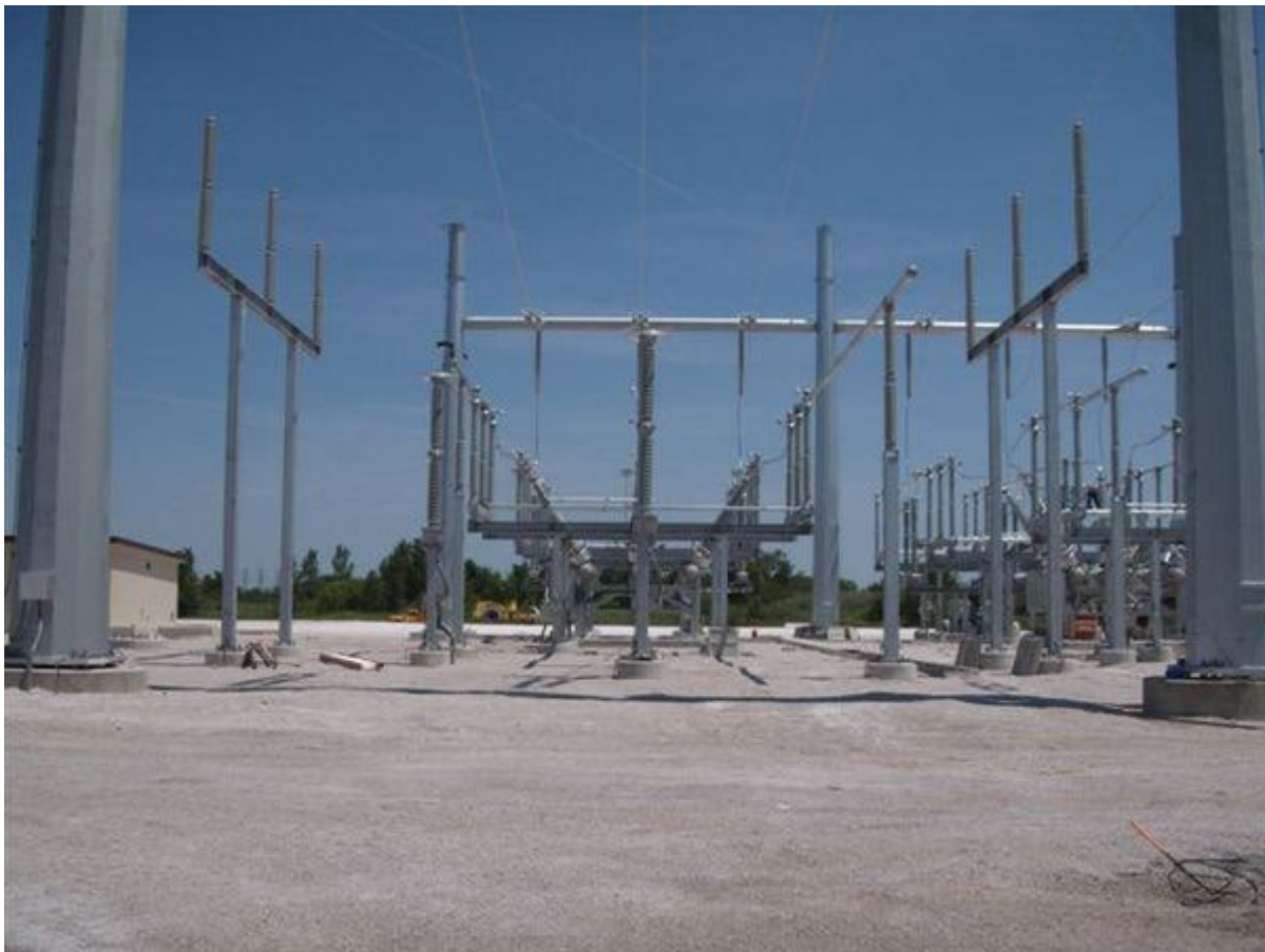
Figure (7) Example of Steel Structures within a Substation 7
