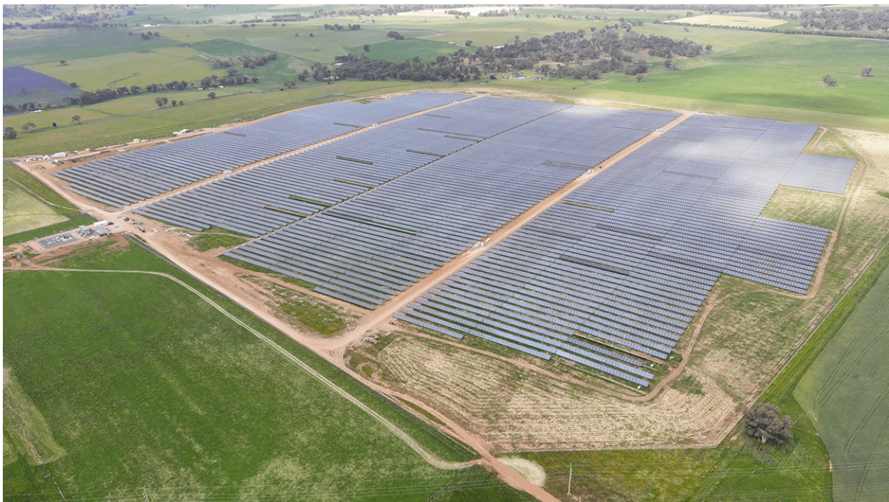
Figure (3) Solar Modules Installed on Farmland 3
