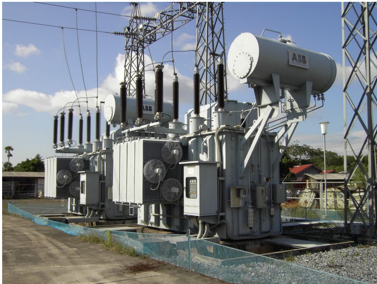
Figure (6) Substation Transformer 6
