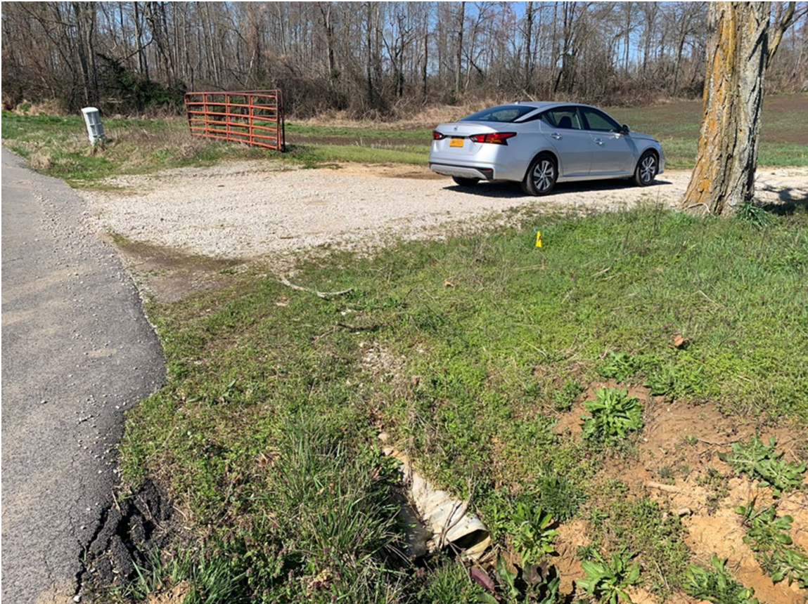
Relatively close by, there is an unpaved access point with a culvert on the eastern side of the road at 37°39'15.4"N 85°58'56.3"W .
