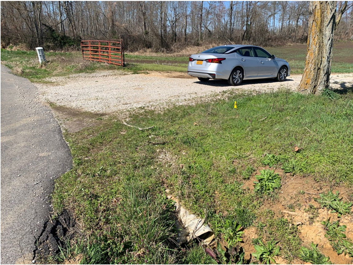
Relatively close by, there is an unpaved access point with a culvert on the eastern side of the road at 37°39'15.4"N 85°58'56.3"W .
