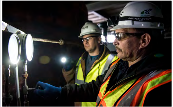
Brent Wasson, left, and Cliff Harmon discuss work being done during the Dale Station demolition.
