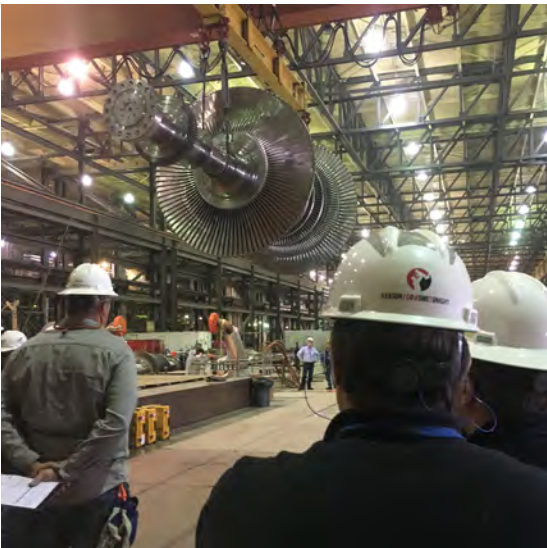
Near the end of the largest outage in EKPC history, workers lift the Unit #4 turbine back into place.
