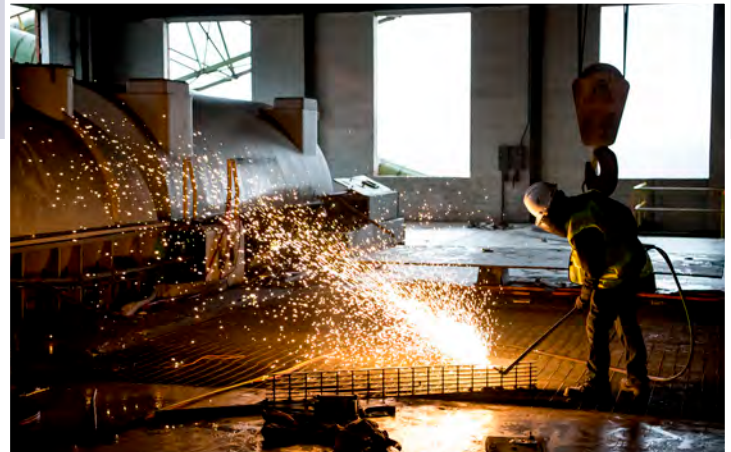
The Dale Station demolition leveled the footprint of EKPC's first power plant.
