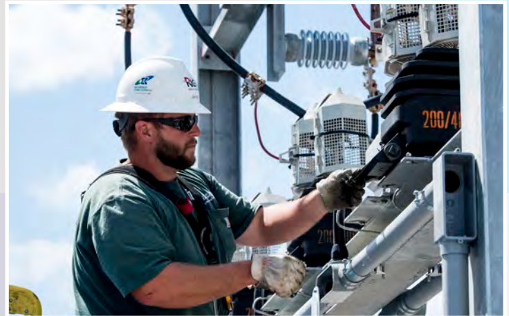
Construction Technician Zach Kelley works on the Hunt Switching Station in rural Clark County.
