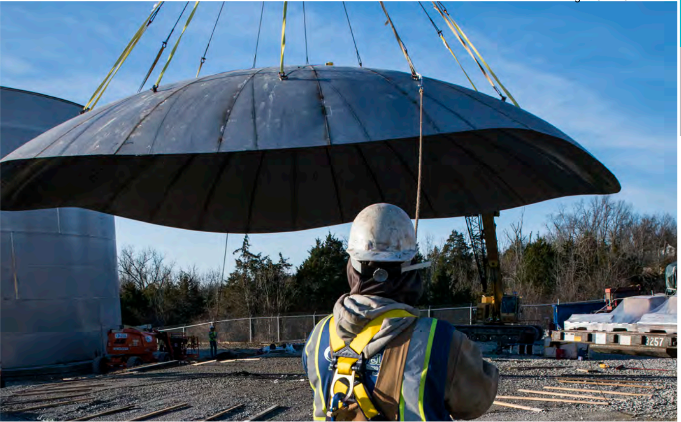
Workers lift the massive top of a new diesel fuel tank at Bluegrass Station.
