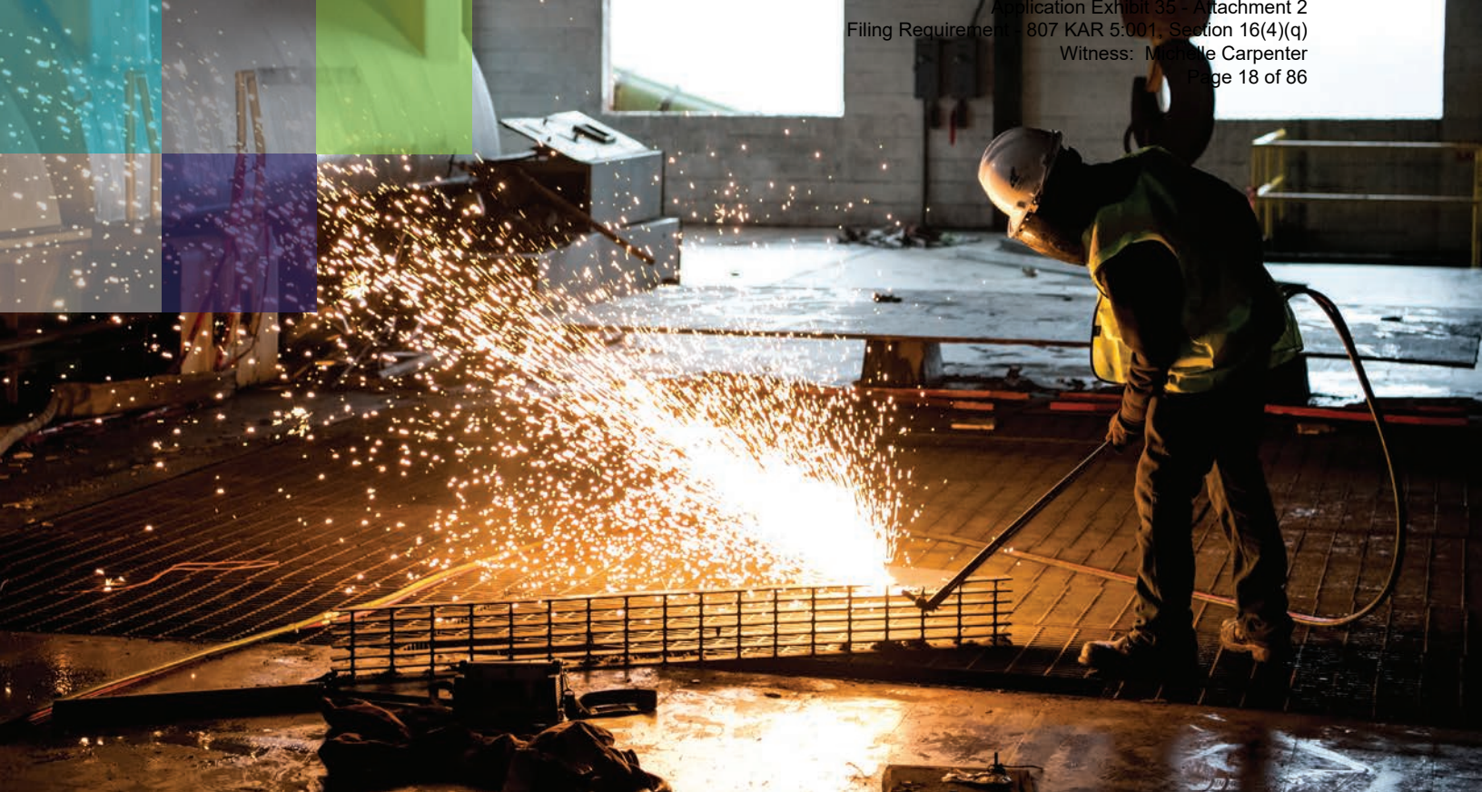
A worker helps in the initial phase of a demolition project to remove the powerhouse and stacks at Dale Station, EKPC's first power plant.
