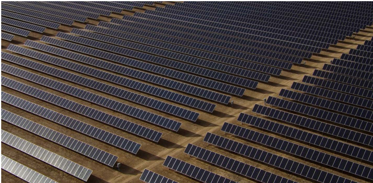
Figure 24-1 — Solar Photovoltaic Project
