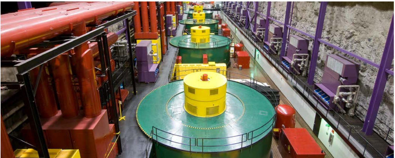
Figure 17-3 — Typical Hydroelectric Power Turbine Hall
