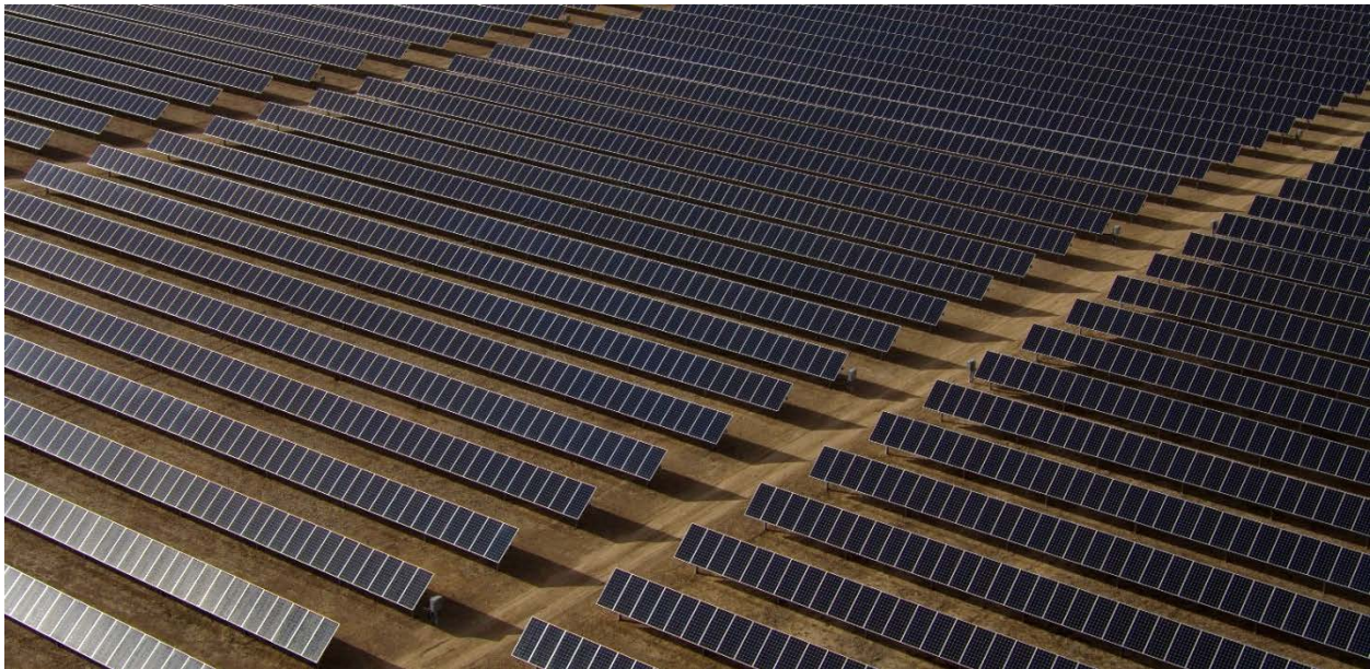
Figure 24-1 — Solar Photovoltaic Project
