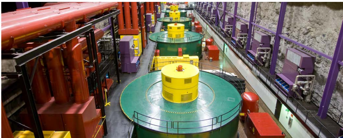
Figure 17-3 — Typical Hydroelectric Power Turbine Hall
