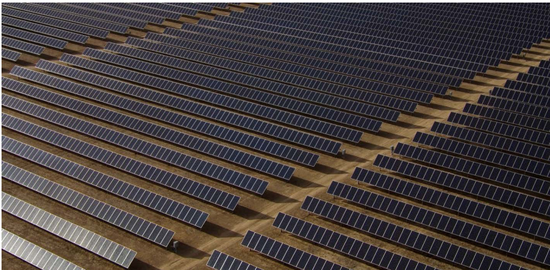
Figure 24-1 — Solar Photovoltaic Project
