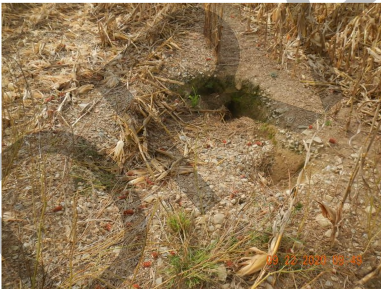
Figure 12: View of feature F-63, reopened throat that was filled with soil and gravel.
