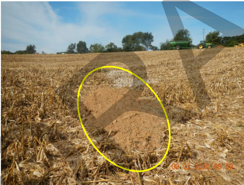
Figure 16: View of feature F-64, small, gently sloped cover subsidence with an apparent fresh soil and gravel filled open throat.
