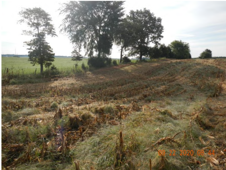
Figure 17: Feature F-53: Small, gentle sloped cover subsidence with no open throat observed.
