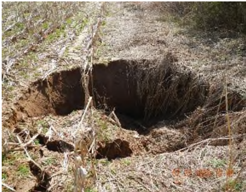
Figure 10: View of feature F-18 a sinkhole with open throat and approximate dimension of 10 feet long, 10 feet wide, and 8 feet deep
