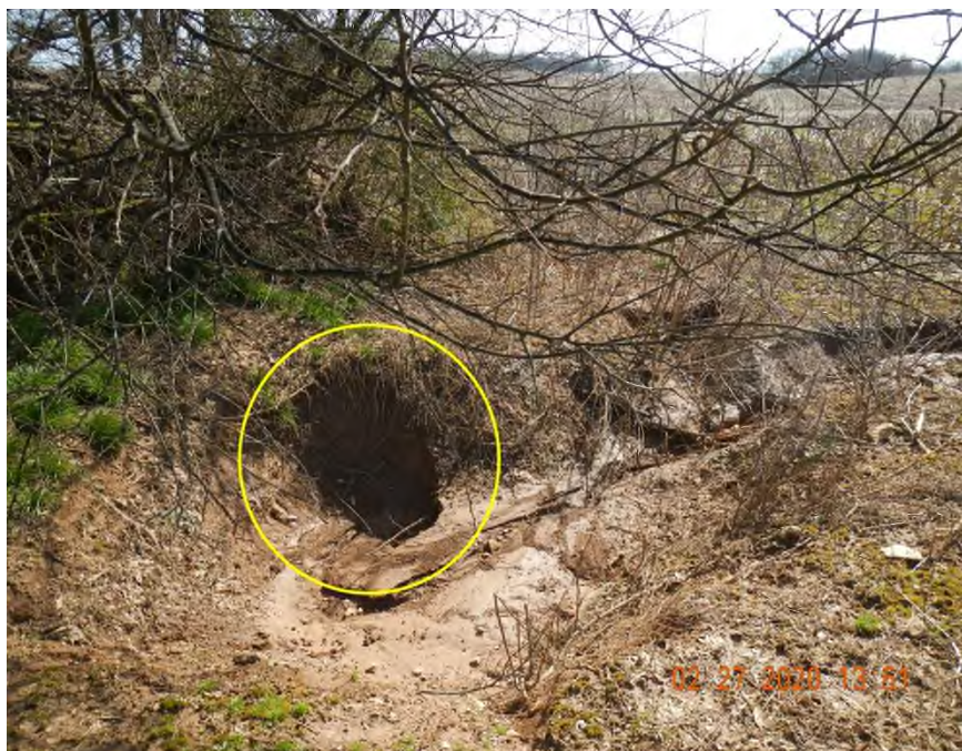
Figure 14: View of feature F-26 a vegetated sinkhole with open throat with an erosion ditch heavily eroded and bare of vegetation.
