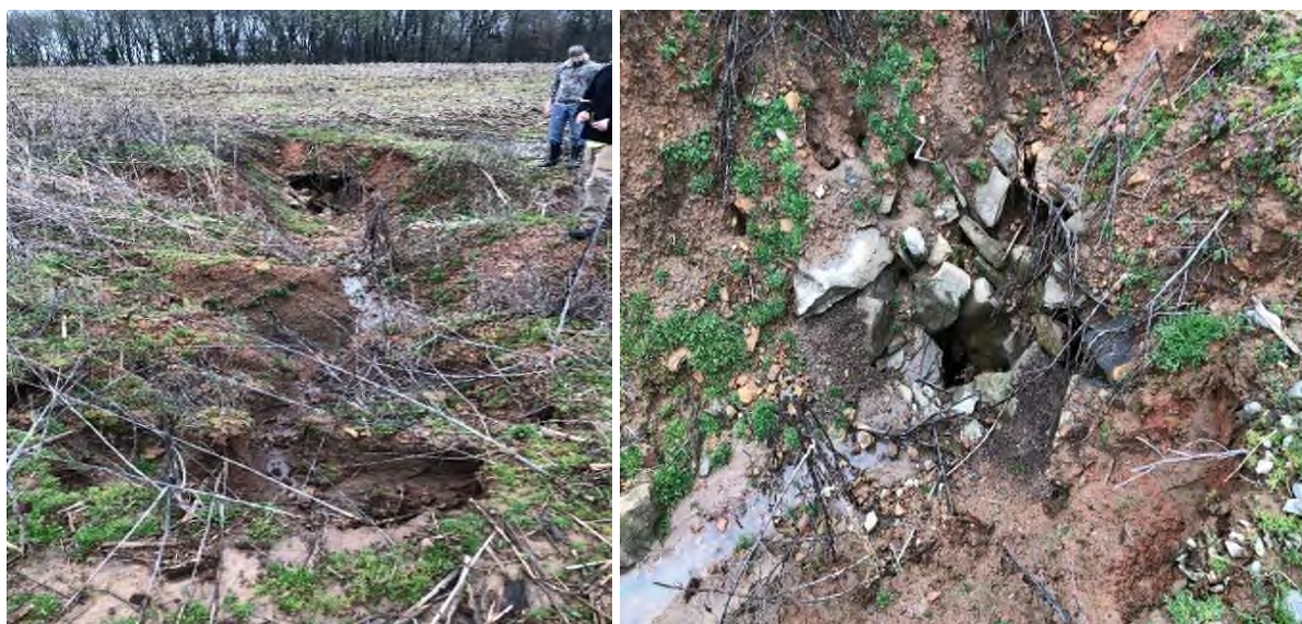
Figure 19, 20, and 21: View of feature F-39 a sinkhole with open throat and surface water draining into subsurface
