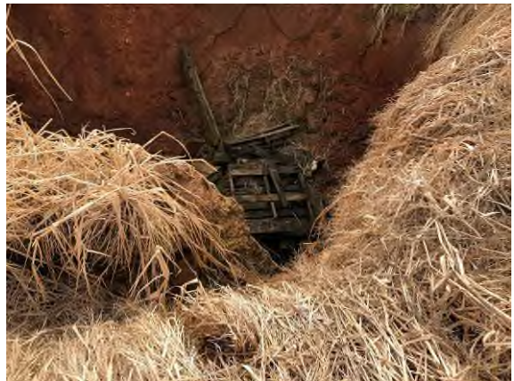
Photo #30 View of southwestern portion of site, and debris in sinkhole - facing south.
