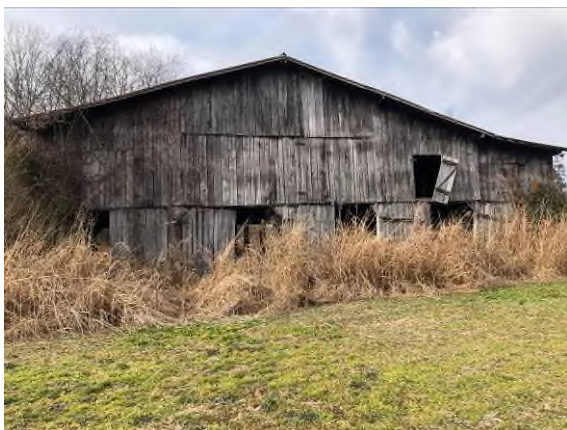
Photo #11 View of southeastern portion of site, and large barn - facing west.
