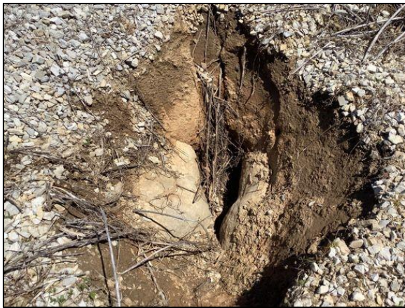
Soil/rock = 2 (failed backfill)
