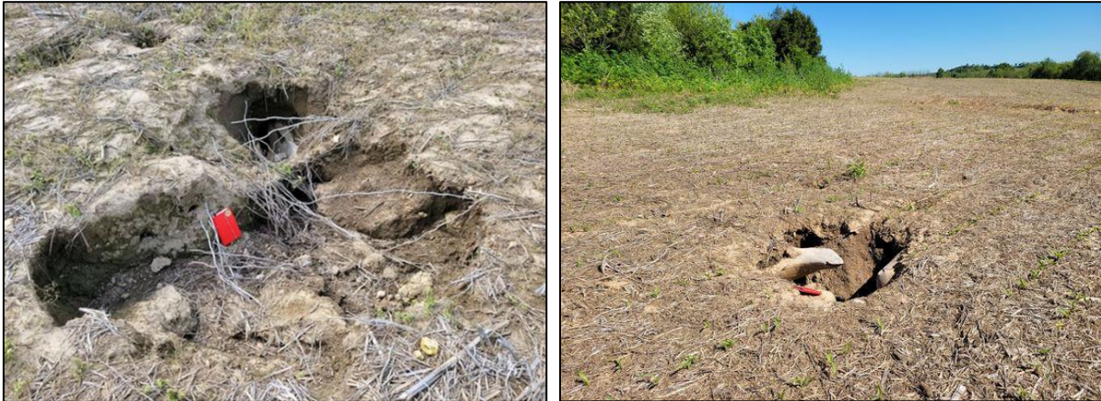
Image 3. Examples of soil piping structures and open throats which are newly developed and indicate that growth and widening of these features is likely.
