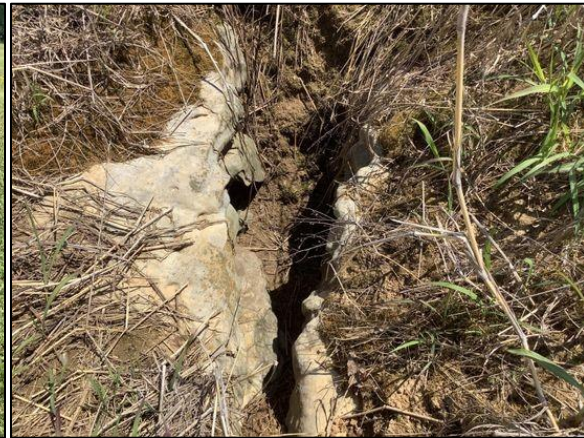
Minor Soil Raveling = 1
