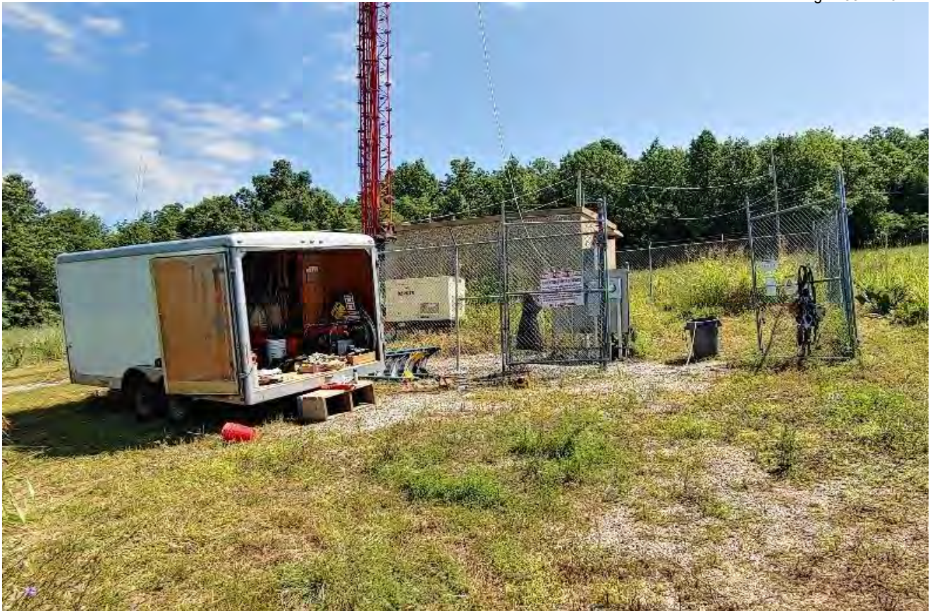
Photo 7: AT&T cell tower and generator. (Parcel 12)
