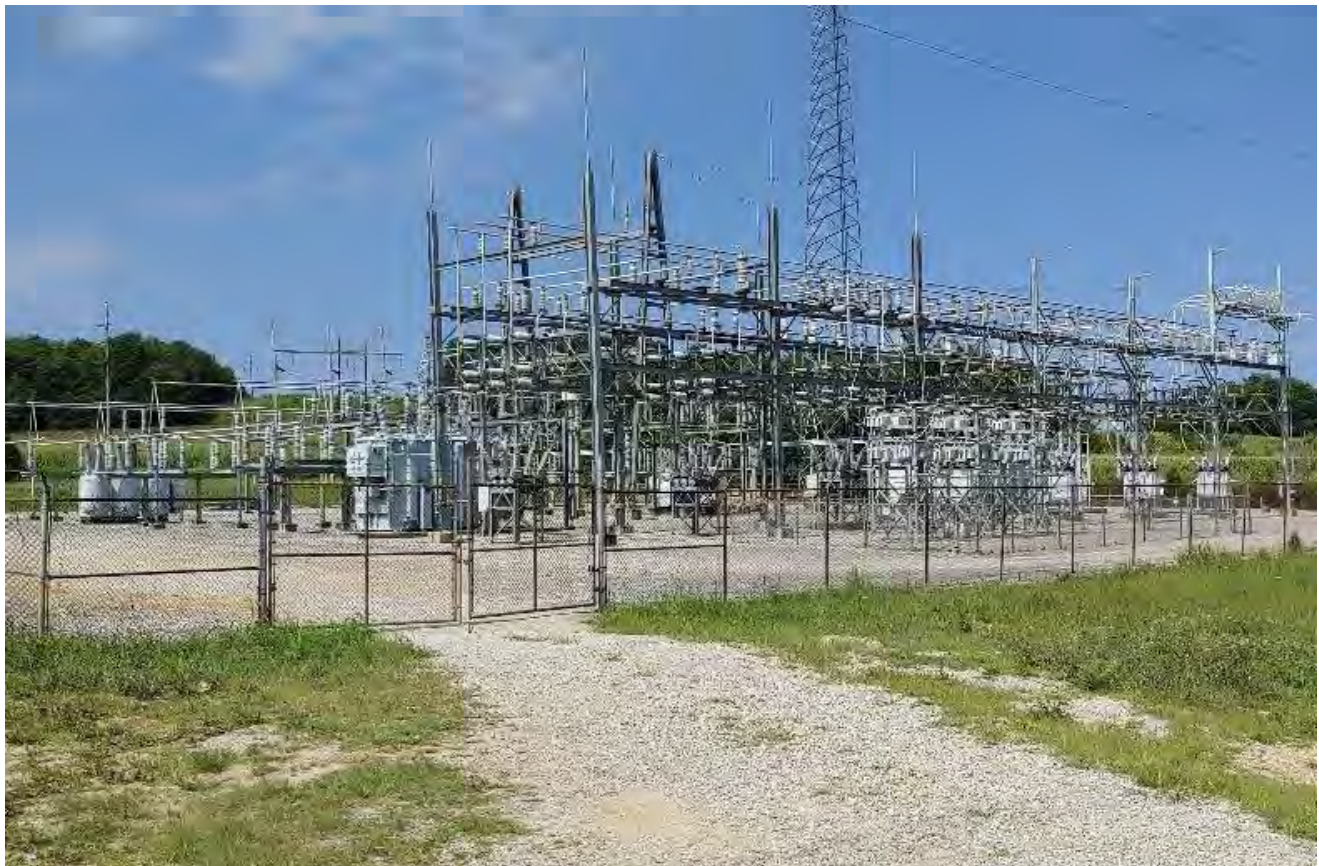
Photo 12: Substation on adjoining property southwest of Parcel 47.
