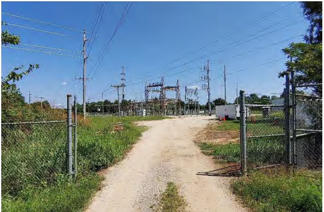
Photo 6: Substation on adjoining property east of Parcel 6.
