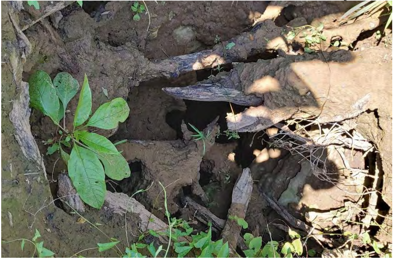
Photo 5: Additional view of the sink hole. (Parcel 6)
