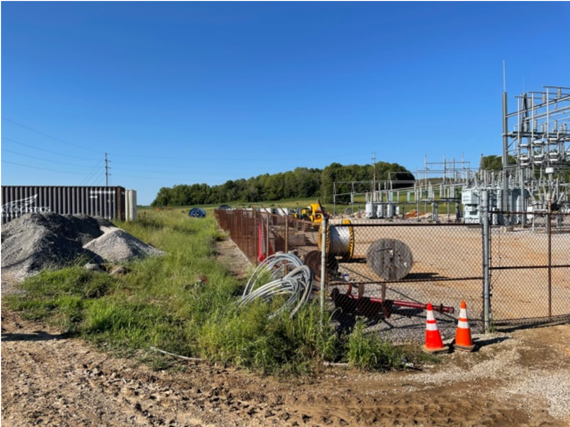
Figure C-7. Existing Meade Substation and Area to Southwest Where New Green River Substation Transformer Would be Built
