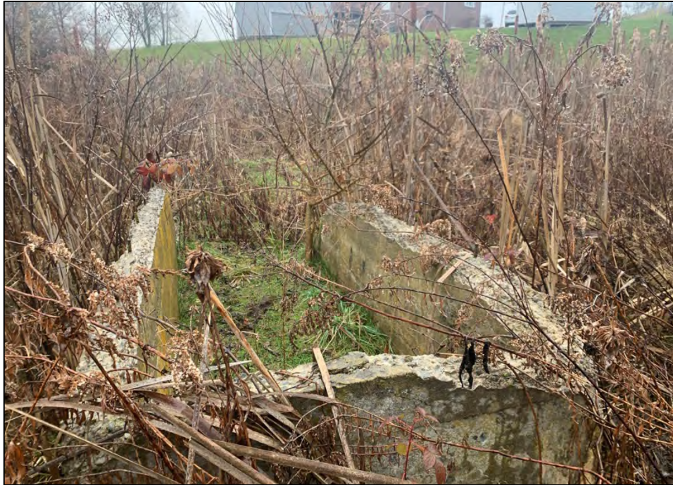
Photo 13: View of typical concrete structure throughout the subject property. View from northeast corner of the Site, facing northeast.
