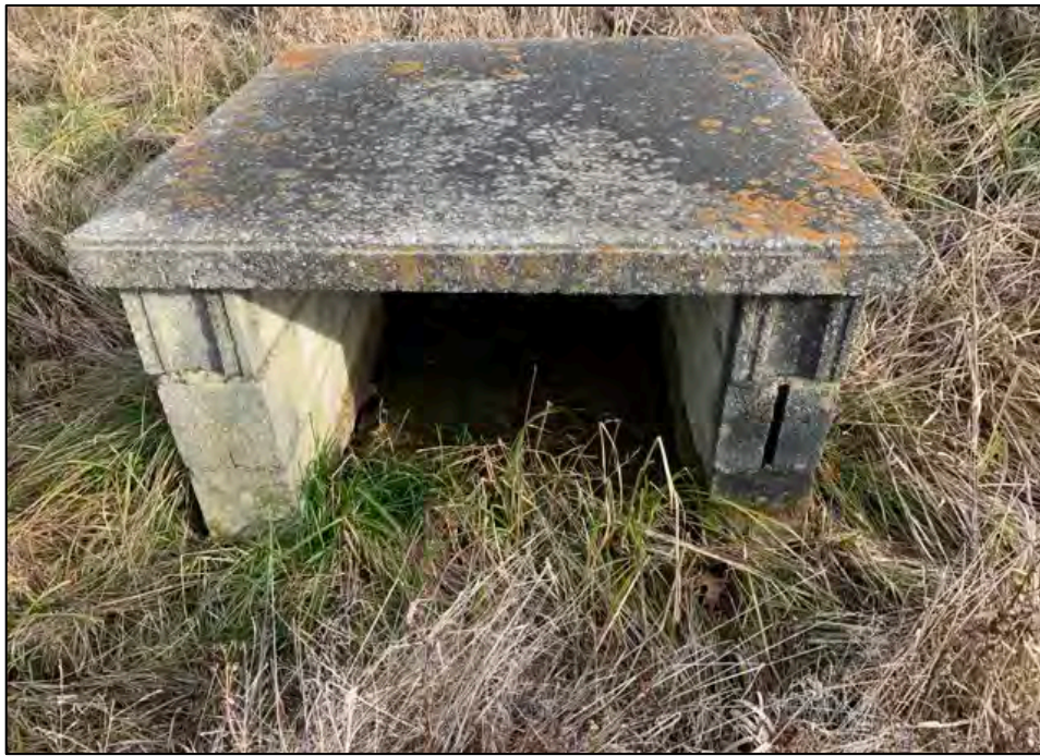
Photo 11: View of cinder block and concrete structure within the subject property. View from northwestern portion of the Site, facing east.
