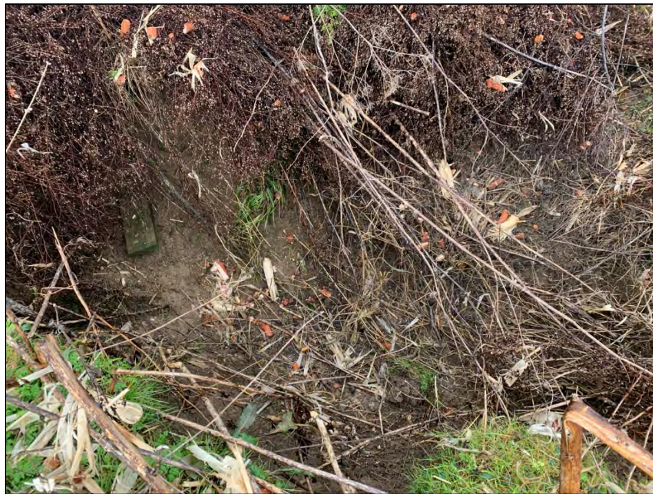
Photo 14: View of Channel 2E widening and hole where system goes underground. View from the end of Channel 2E in the southeastern portion of the Site.
