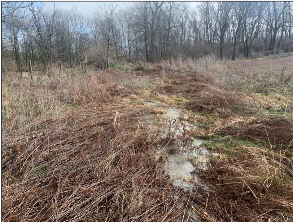
Photo 59: Typical view of Feature 23 from its southern end, facing north. Photo taken on March 17, 2021.
