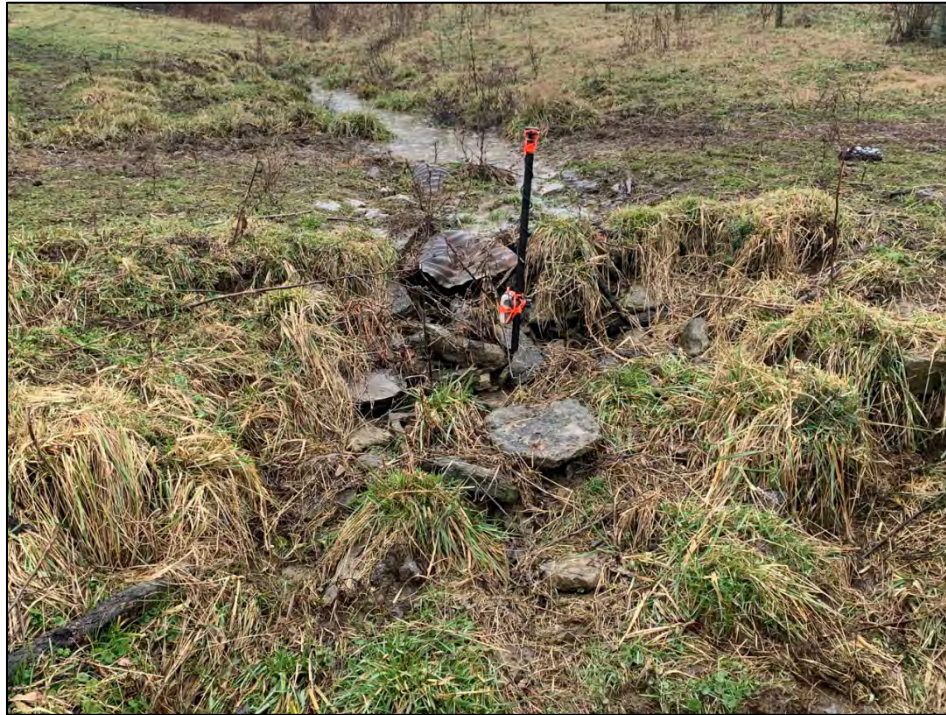
Photo 38: View of Channel 22 ending at a pipe. View from the terrace of Channel 20, facing west.
