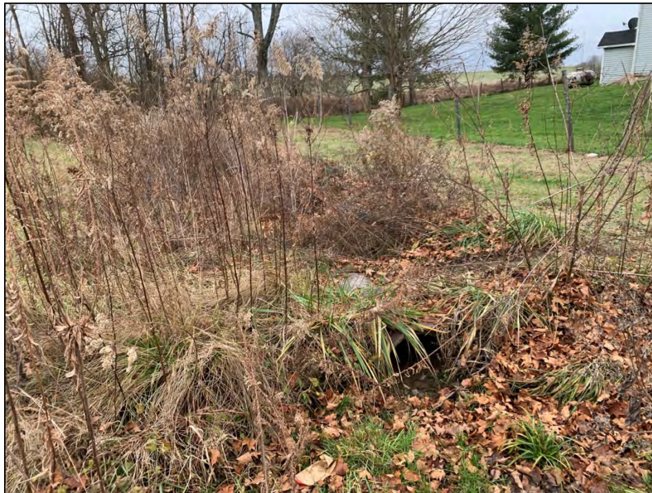
Photo 52: View of culvert connecting Feature 9 to Channel 8. View from the southern portion of Feature 9, facing southeast.
