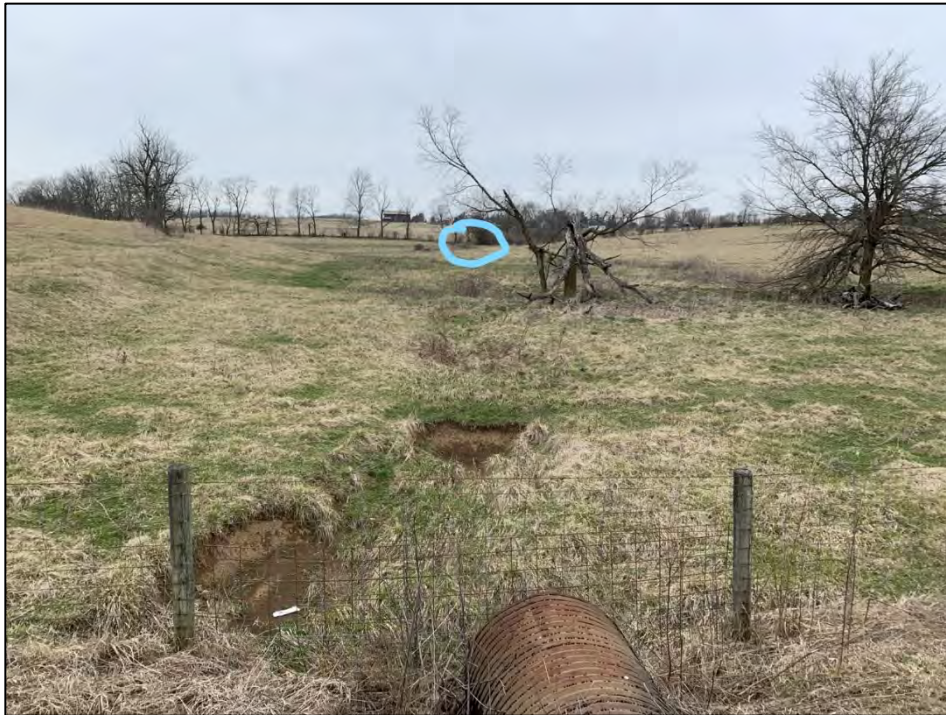
Photo 53: View of offsite upland drainage downgradient from Channels 1, 2E, and 6. View from Convict Pike facing west towards Channel 1 circled in blue. Photo taken on March 17, 2021.
