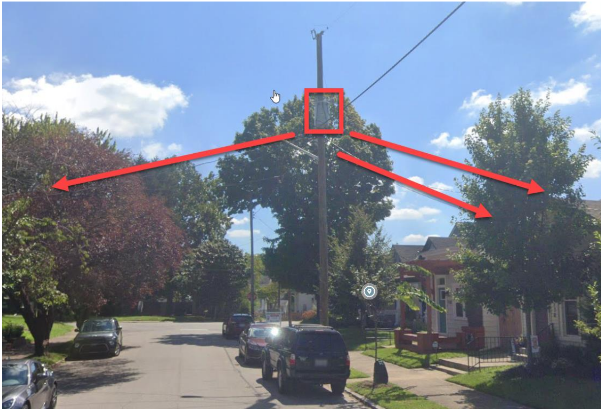
Figure 1 – Failing service transformer Identified via AMI telemetry.
