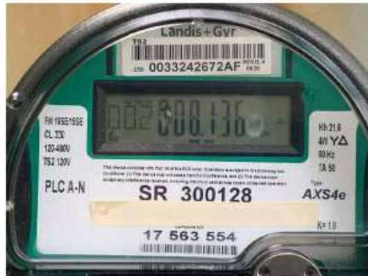
WWTP Electrical Meter
