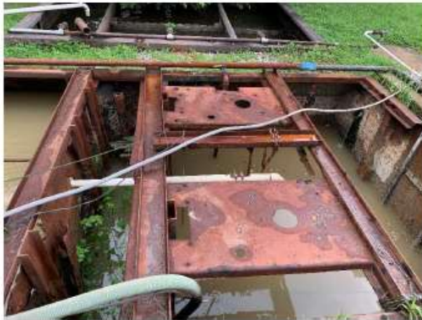
EQ Basin, Portable Pump Discharge, Digester, Miscellaneous Electrical Cables
