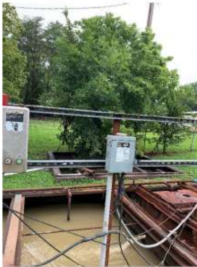
Electrical Boxes and Electrical Cabling
