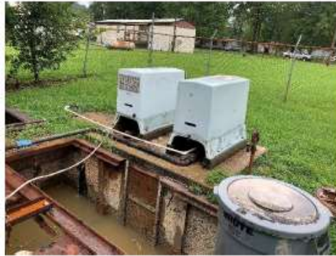
Blowers, EQ Basin, and Electrical Cables
