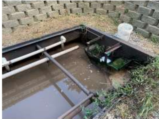
Manually Cleaned Bar Screen
