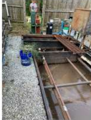
Aeration Tank, Clarifier, Contact Tank
