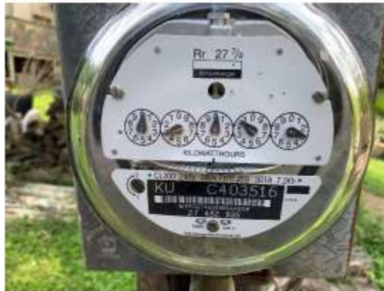
WWTP Electrical Meter
