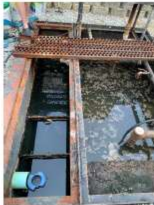
Clarifier and Contact Tank
