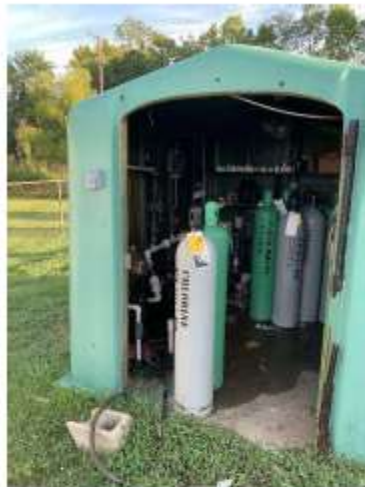
Gaseous Chlorine Storage
