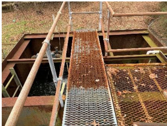
9 10 Extensive rust on walkways, handrails and tank structure.
