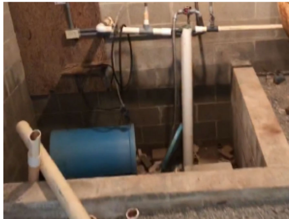
13 14 Out-of-service well with freeze-damaged piping.
