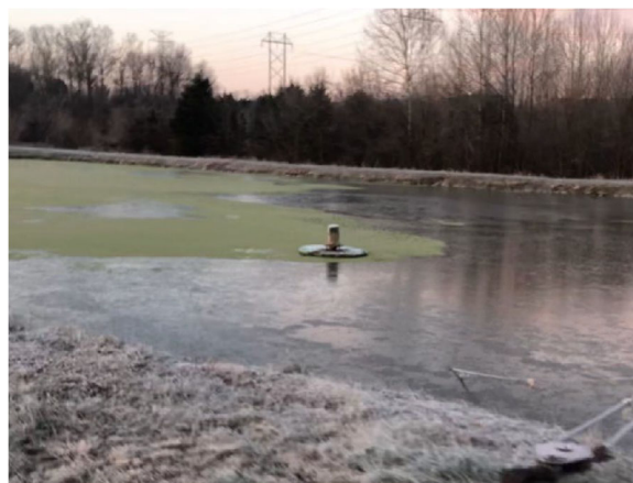
10 11 12 Nonfunctional blower in lagoon. 13
