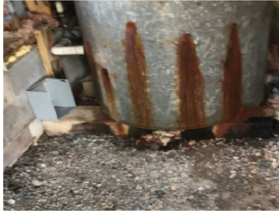
Rust damage and leaking hydropneumatic tank.
