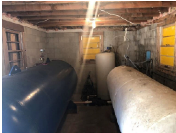
Storage tanks and chlorine dosage in the same room with exposed wiring and no finish carpentry.
