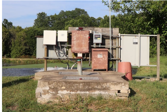
Mission remote monitoring installed
