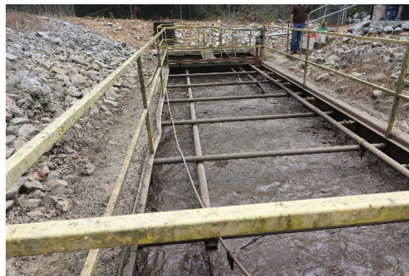
17 18 Notable corrosion on steel equipment and staining from regular flooding
