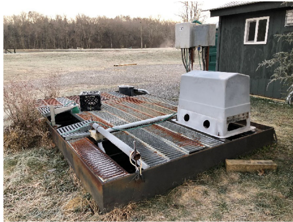
Chlorine system with post aeration.
