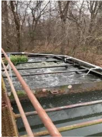
6 7 Vegetation growing on top of the wastewater treatment facility.
