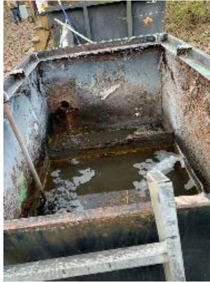
Severely deteriorated contact chamber.
