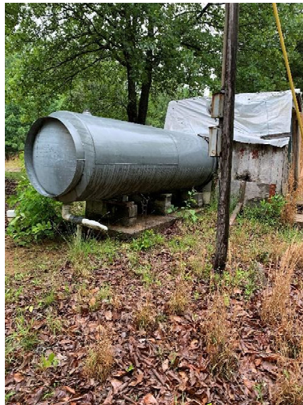
4 5 Unpainted hydropneumatic storage tank.
