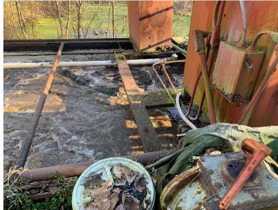
Corrosion of steel tankage structures.
