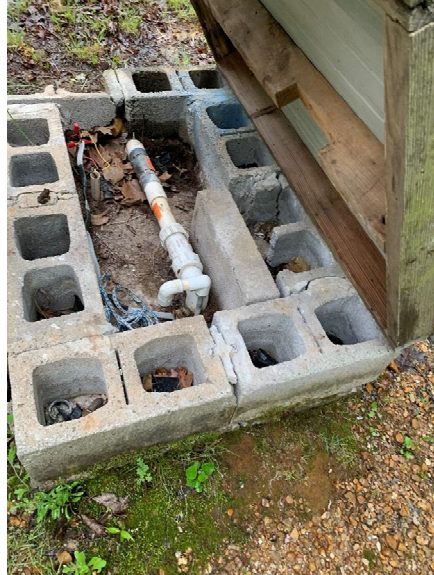
1 2 Deteriorating cinder block containment for well head covered in mouse and toad droppings with vermin 3 infiltration.
