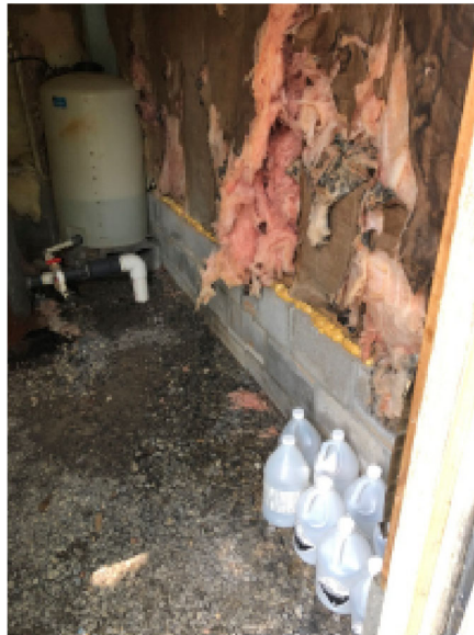
Interior of functional well house, dirty and dilapidated.
