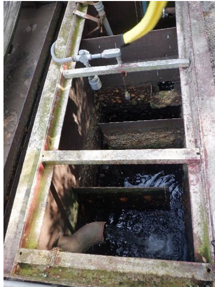
Corrosion of steel components.
