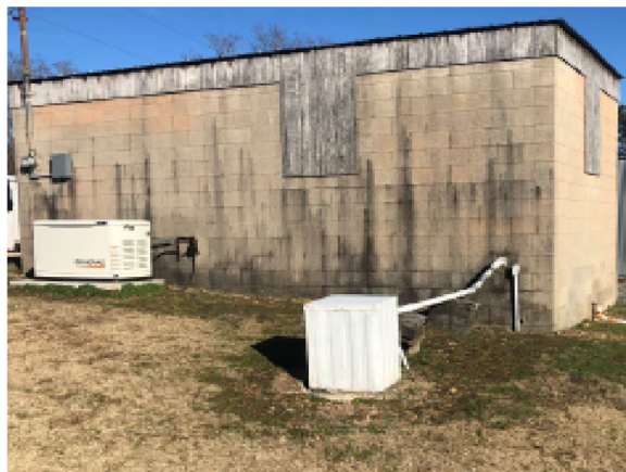
No Fencing or proper access to the facility.
