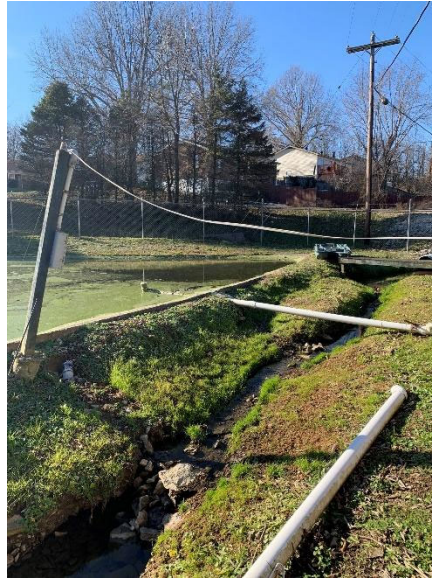
Stormwater erosion on site.
