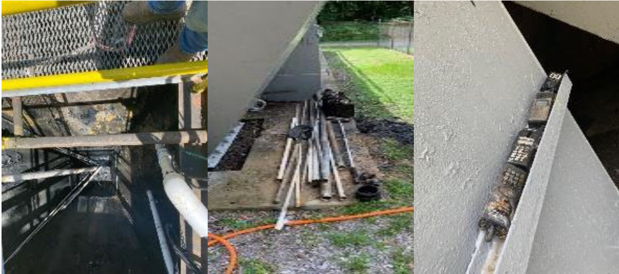
Debris in bottom of clarifier and debris after removal from clarifier.
