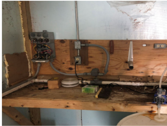
Exposed wiring and ineffective chlorine dosage equipment.
