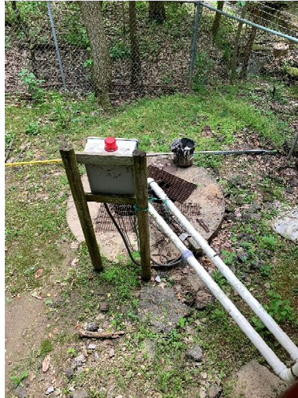
Influent Lift Station lines improperly installed
