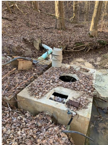
Failed contact chamber and improperly improvised effluent structure.
