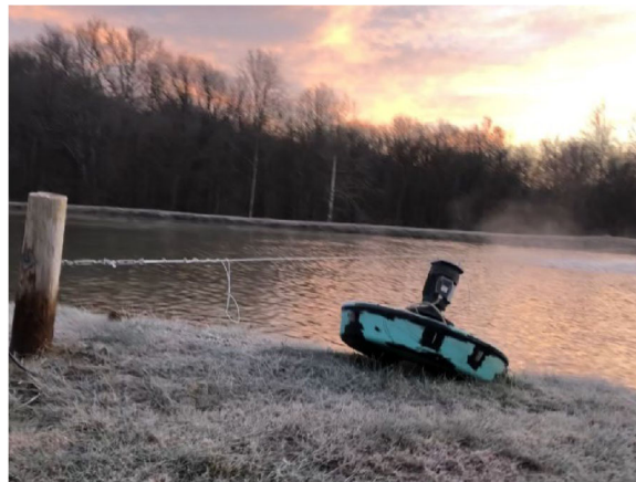
8 9 Inactive blower on lagoon berm.
