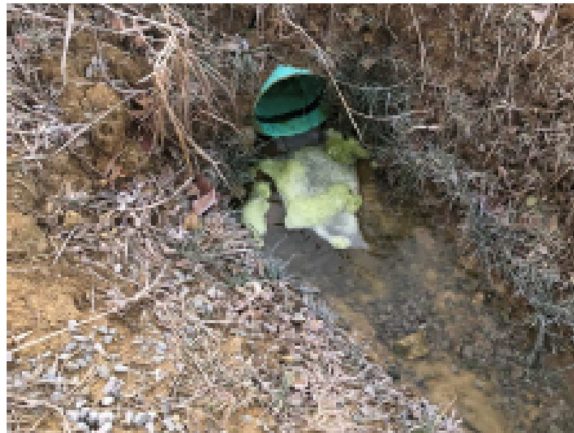
Discharge pipe feeding into open dirt channel.
