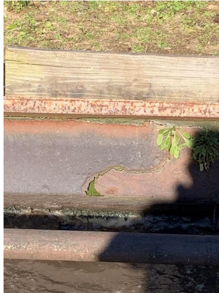
Corrosion of steel tank structure.
