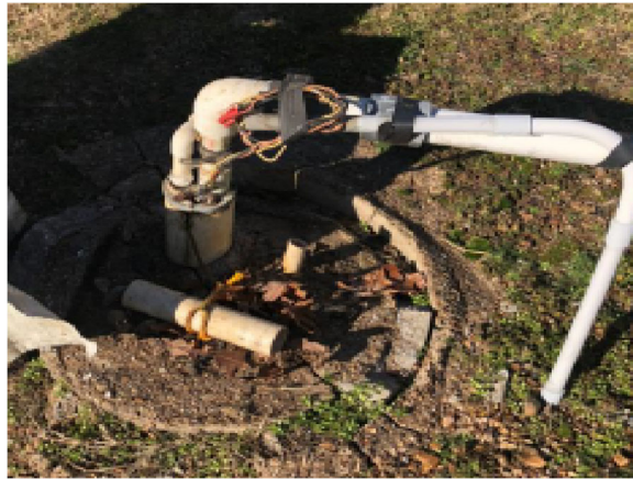
Well head with exposed wiring.
