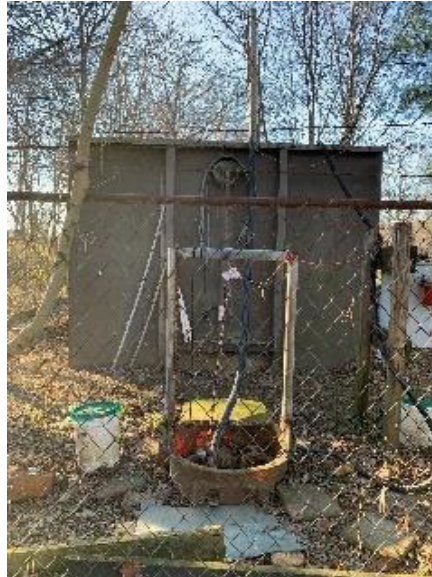
Influent lift station with improvised pumping design into treatment plant.
