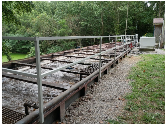
11 Vegetation removed, steel repairs in place, blower housings repaired, and debris removed. New 12 RAS (sludge return) visible in shot, repainted handrails. 13 14
