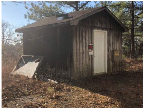
12 Rotting wood paneling on the existing well house. 13 14
