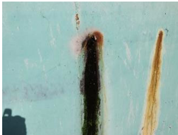
6 7 Steel tankage with rusted holes stuffed with sticks to reduce leakage instead of proper repair
