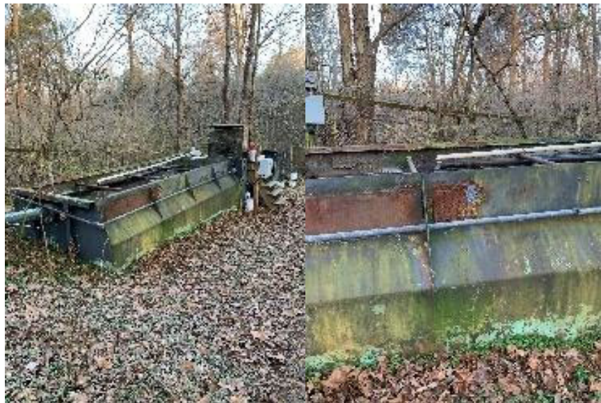
Deterioration of aeration tankage.
