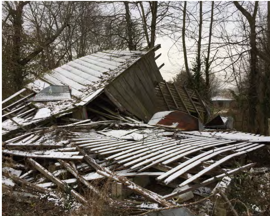
14. A collapsed outbuilding on Parcel 38-20 typical of other collapsed buildings in forested areas throughout the subject site.
