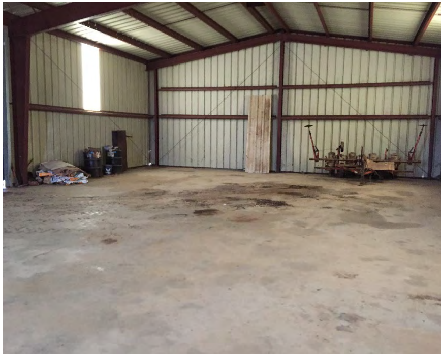
4. Inside the red metal framed barn on Parcel 49-6. The concrete floor was observed to be in good condition with de minimis staining observed.
