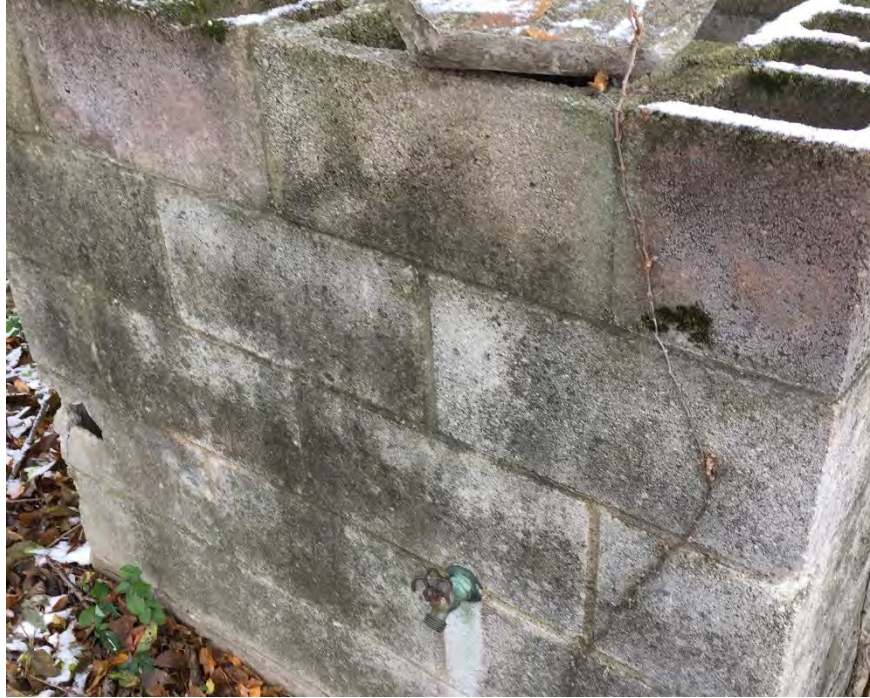
39. A spicket at a concrete block water structure near a pond on Parcel 38-5.
