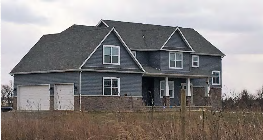
4,255 square foot estate home under construction, adjacent to Portage Solar Farm located in Indiana On-site pond and attached garage (cost estimated at $465,000) April 2018
