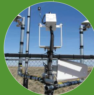
Communications and Technical Equipment
