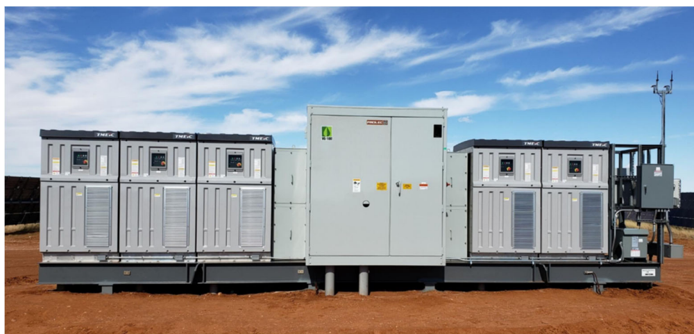
Figure 4 Typical Inverter and Transformer Station
