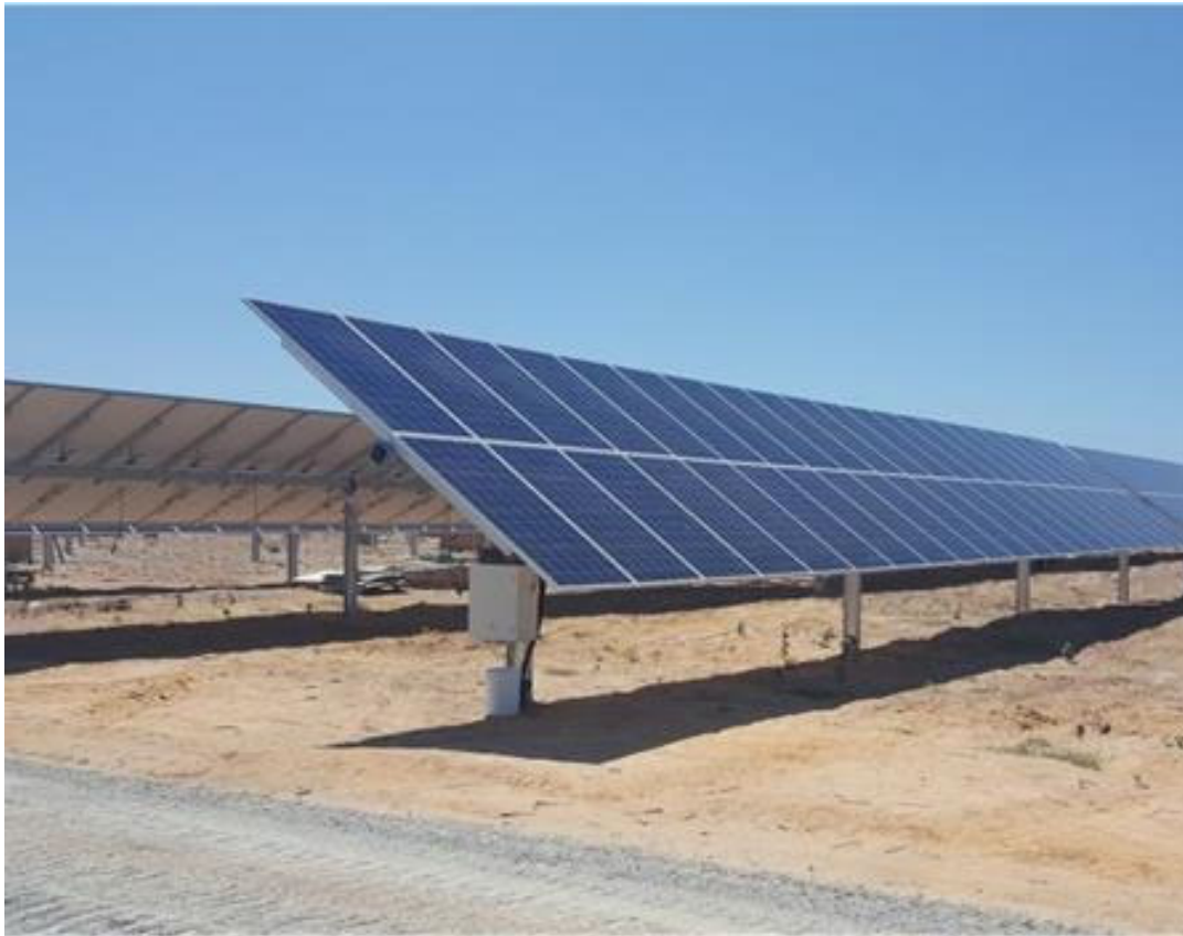
Figure 1B Fixed Tilt Rack System
