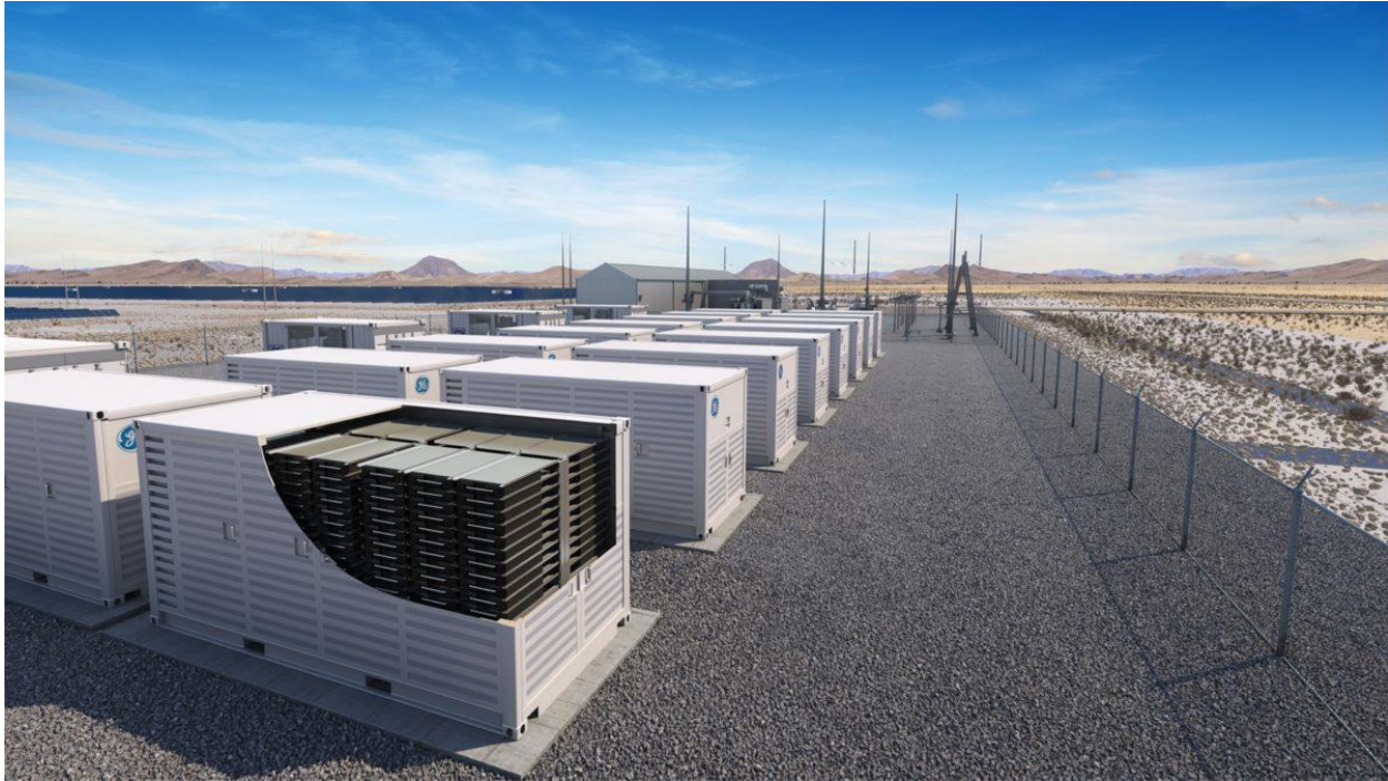
Picture (5) GE Industrial Battery 6
