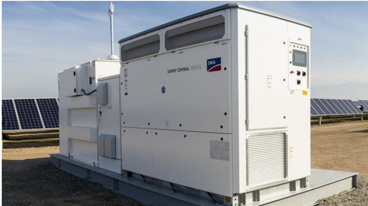
Picture (4) Industrial Solar Inverter 5
