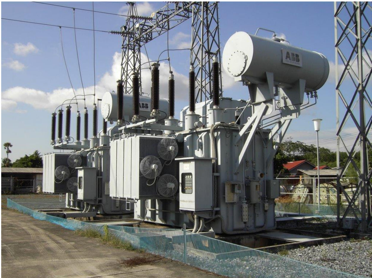
Picture (6) Substation Transformer 7
