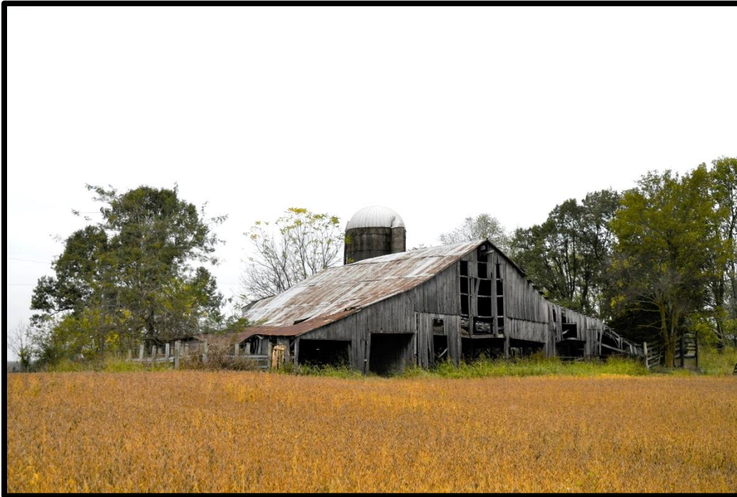
Plate 166. CA-24A and B, Transverse frame barn and Silo, southeast (front) and southwest elevation, looking north.
