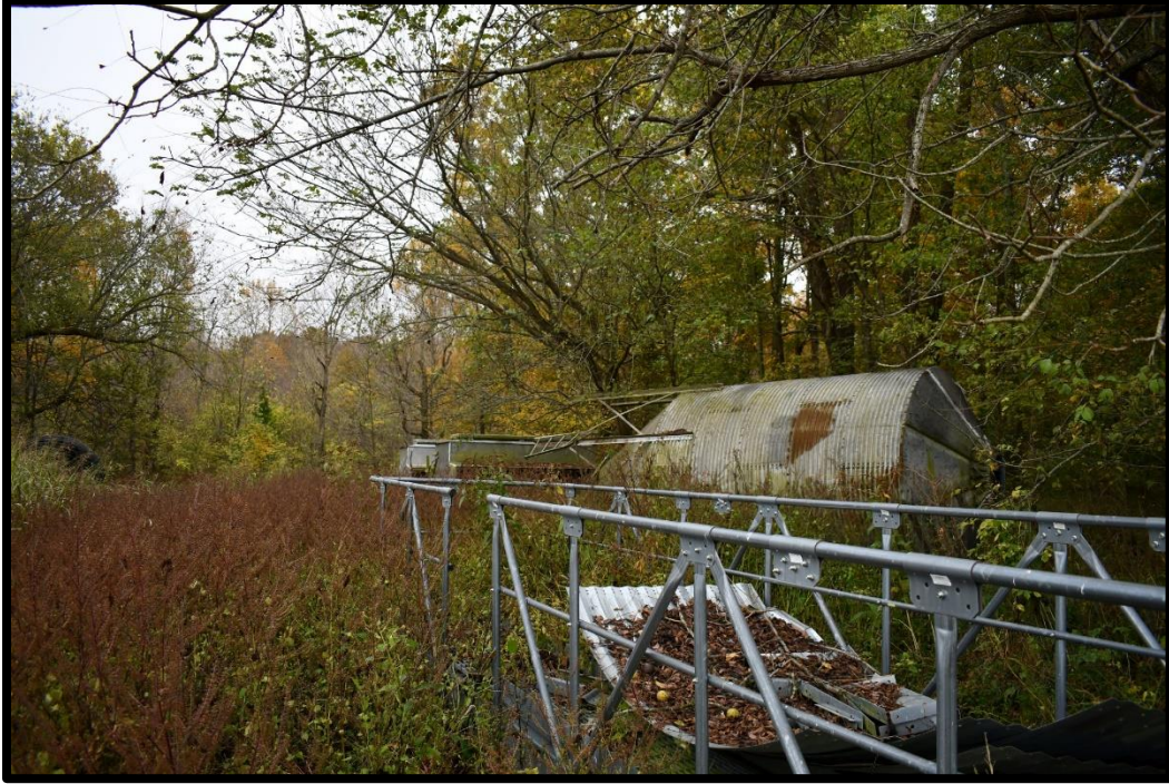
Plate 172. CA-24H, Collapsed Water Tower, looking southeast.
