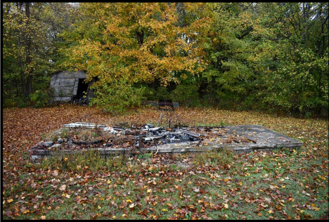
Plate 123. CA-445B, Building Foundation with the shed, CA-445, in background, southeast elevation, looking northwest.
