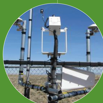
Communications and Technical Equipment
