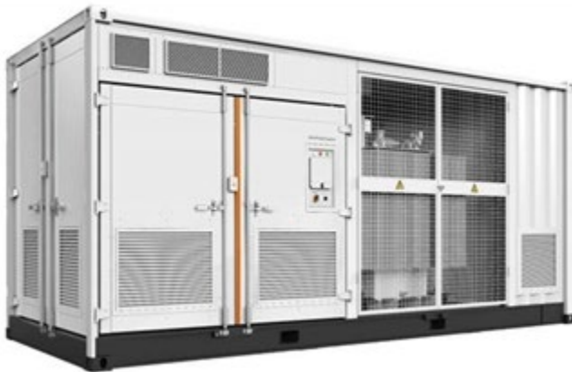
Figure 6 Typical Inverter and Transformer Station
