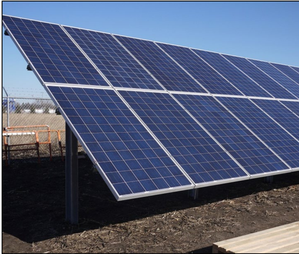
Figure 3 Fixed-Tilt Racking System
