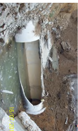
48" Water Main Break
