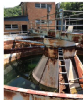
Failed Treatment Clarifier
