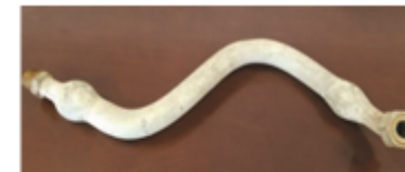
3/4" lead service line
