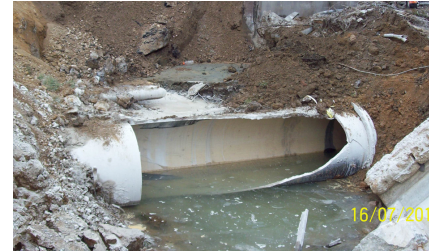
48" Water Main Break
