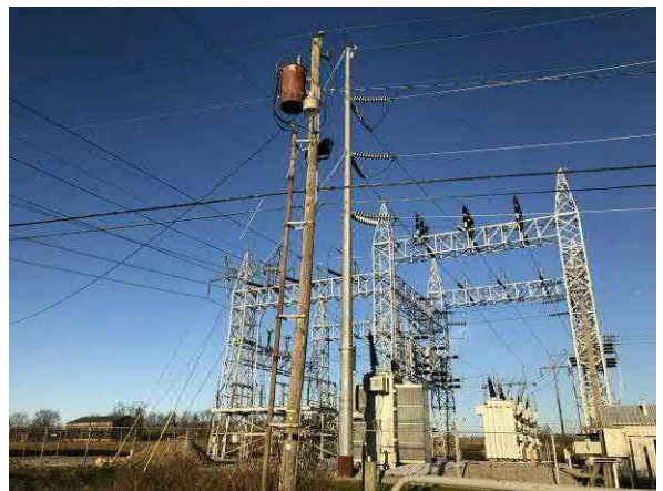
Photo #12 View of electrical substation north of Radio Station Road, adjoining southwest portion of site.
