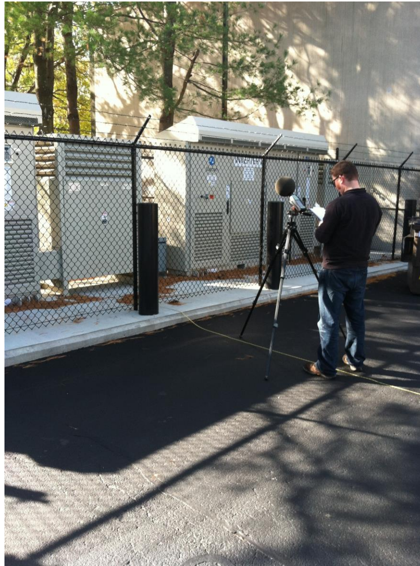
Figure 2. Sound Level Meter on the Axis Perpendicular to the Face of an Inverter at a Solar Photovoltaic (PV) Array
