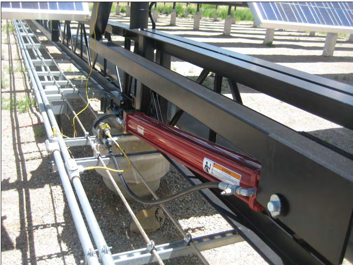
Figure 8: Example of a Tracking Solar PV Installation
