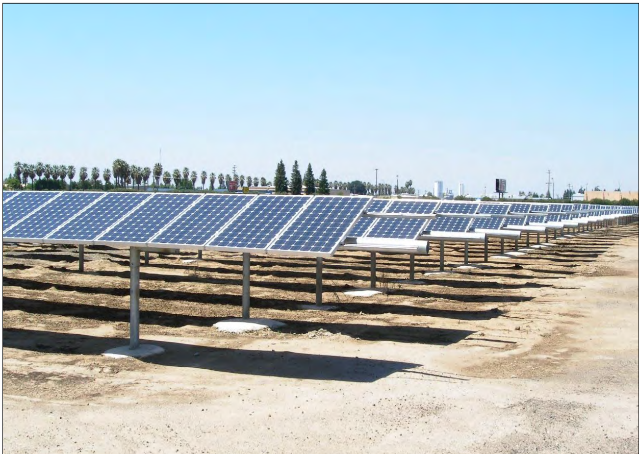
Figure 7: Example of a Ground-Mounted Solar PV Installation
