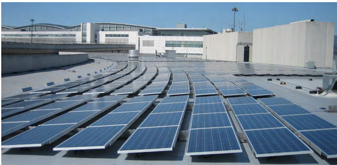
Figure 24: Rooftop Solar Project on San Francisco’s Terminal 3
