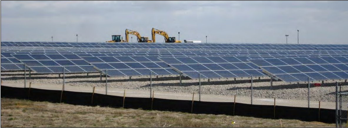
Fixed System at the Fuel Farm Solar Farm
