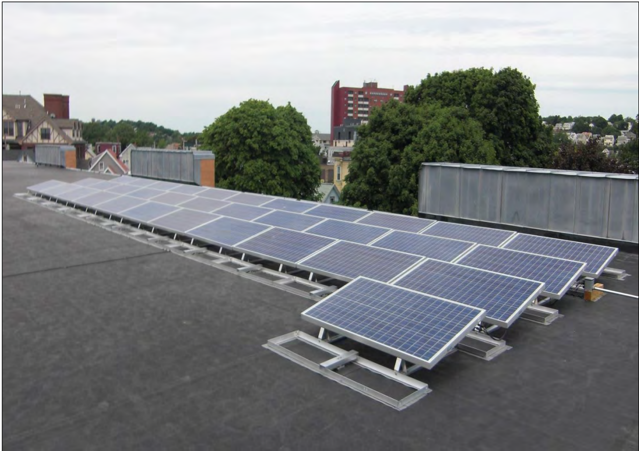
Figure 6: Example of a Roof-Mounted Solar PV System
