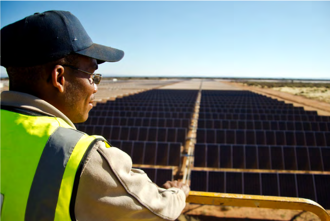
A local worker surveys panels at ACCIONA's Sishen solar farm in South Africa.
