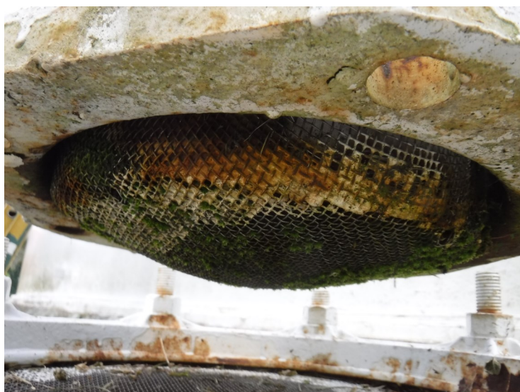
6) The overflow pipe discharge screen partially plugged with debris.
