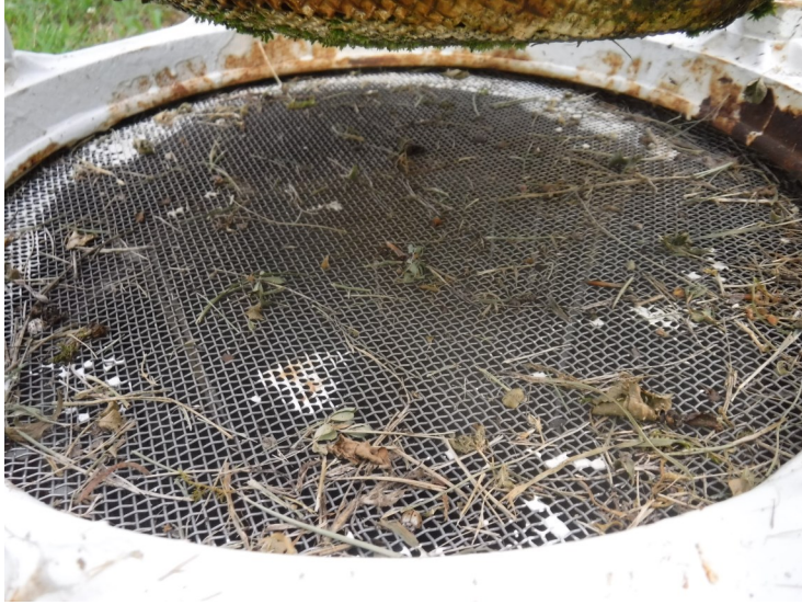
7) Grass clippings covering the drain line screen.
