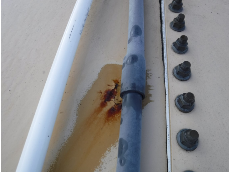
13) Spot lining deterioration on the roof with rust undercutting.
