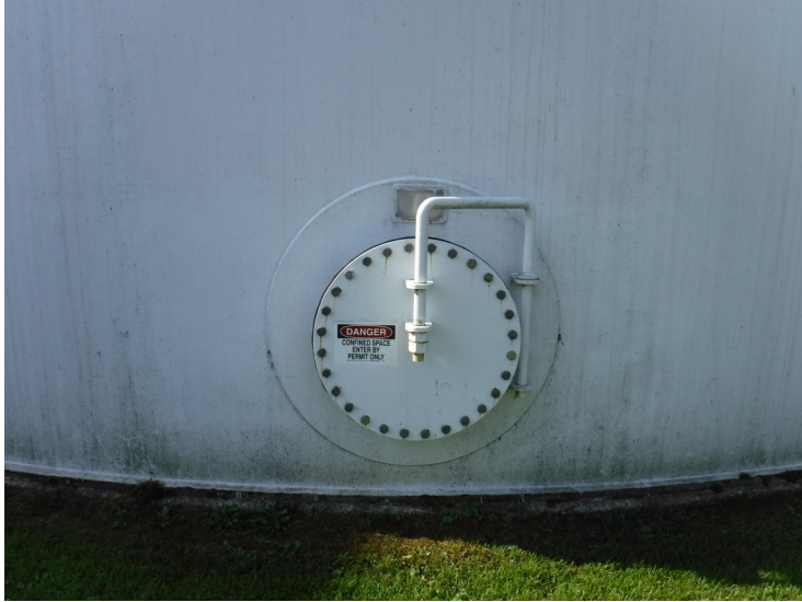
7) Hinged sidewall manway for tank entry.
