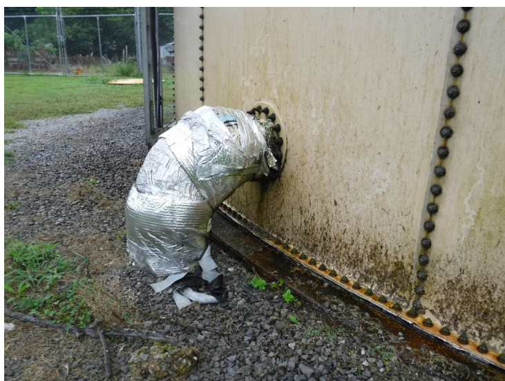
6) The fill pipe is covered with insulation.
