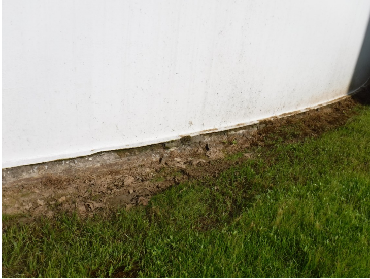
1) Loose and missing grout between the baseplate and foundation.
