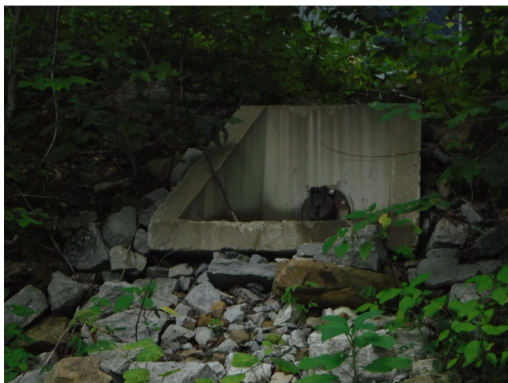
6) The overflow discharges through the side of the hill. The concrete pad is in good condition.
