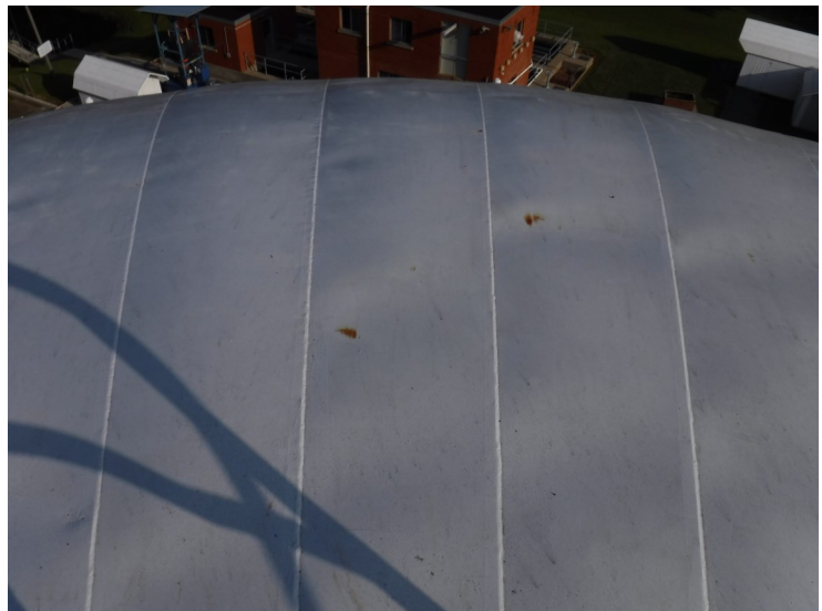
14) Rust bleedthrough on the roof.
