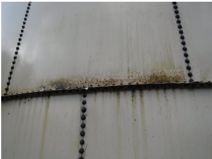
9) Lining deterioration at the bolted flanges.
