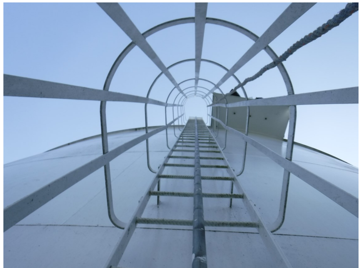
8) Sidewall ladder with rail type fall prevention device.
