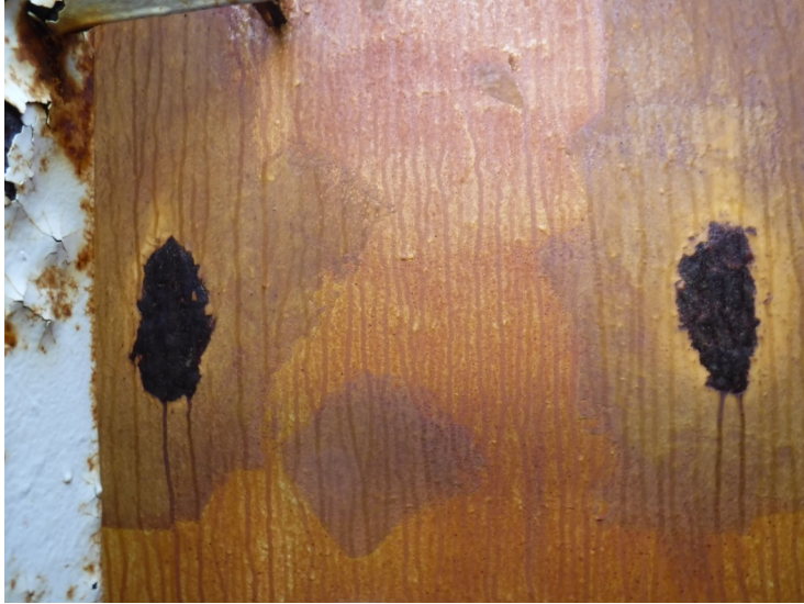
22) Spot coating failures on the upper sidewall.
