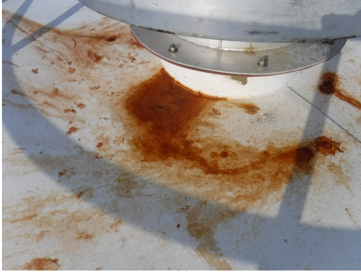
13) Rust staining around the vent neck.
