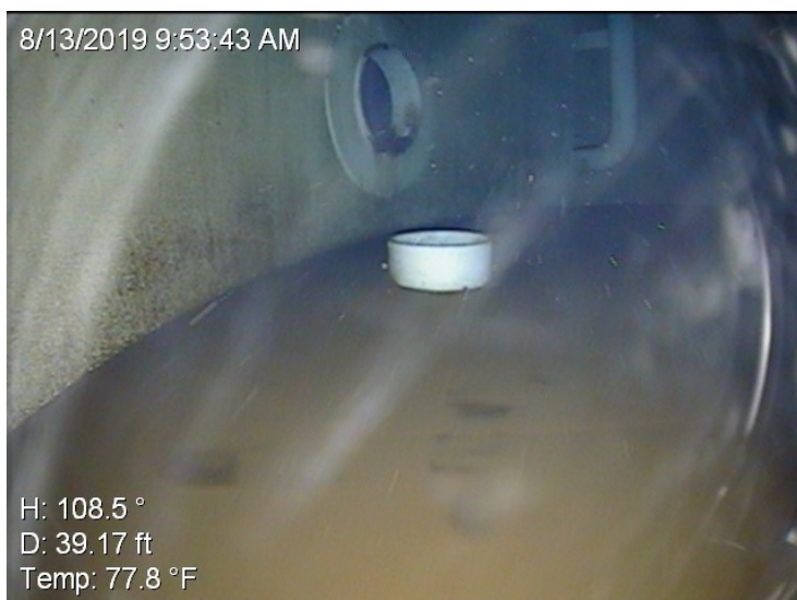
30) The wet interior floor is covered with sediment.
