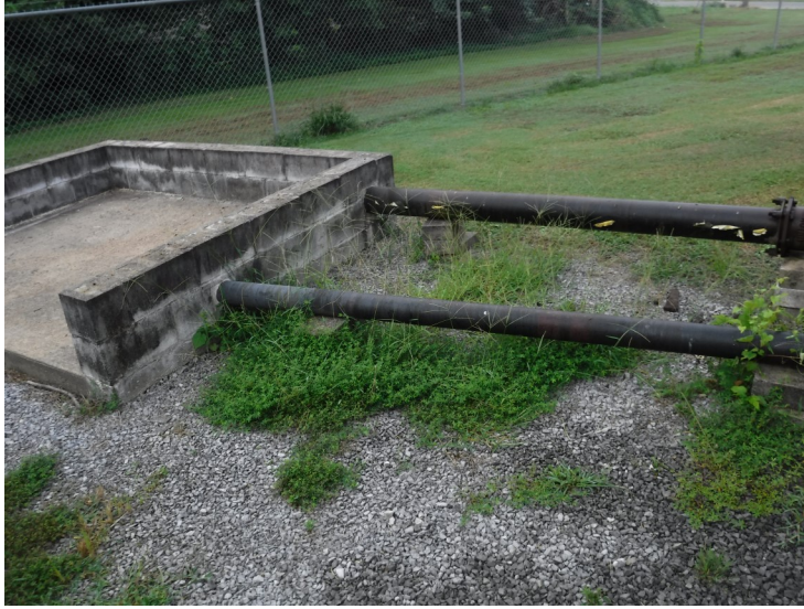
4) Overflow pipe and drain line discharge to a splash pad. The pipe coating is in poor condition.
