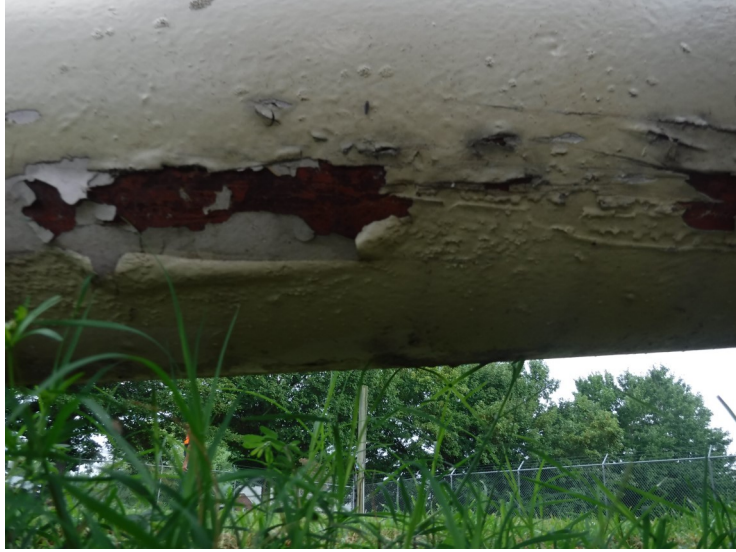
7) Spot coating failures and delamination on the bottom of the overflow pipe.
