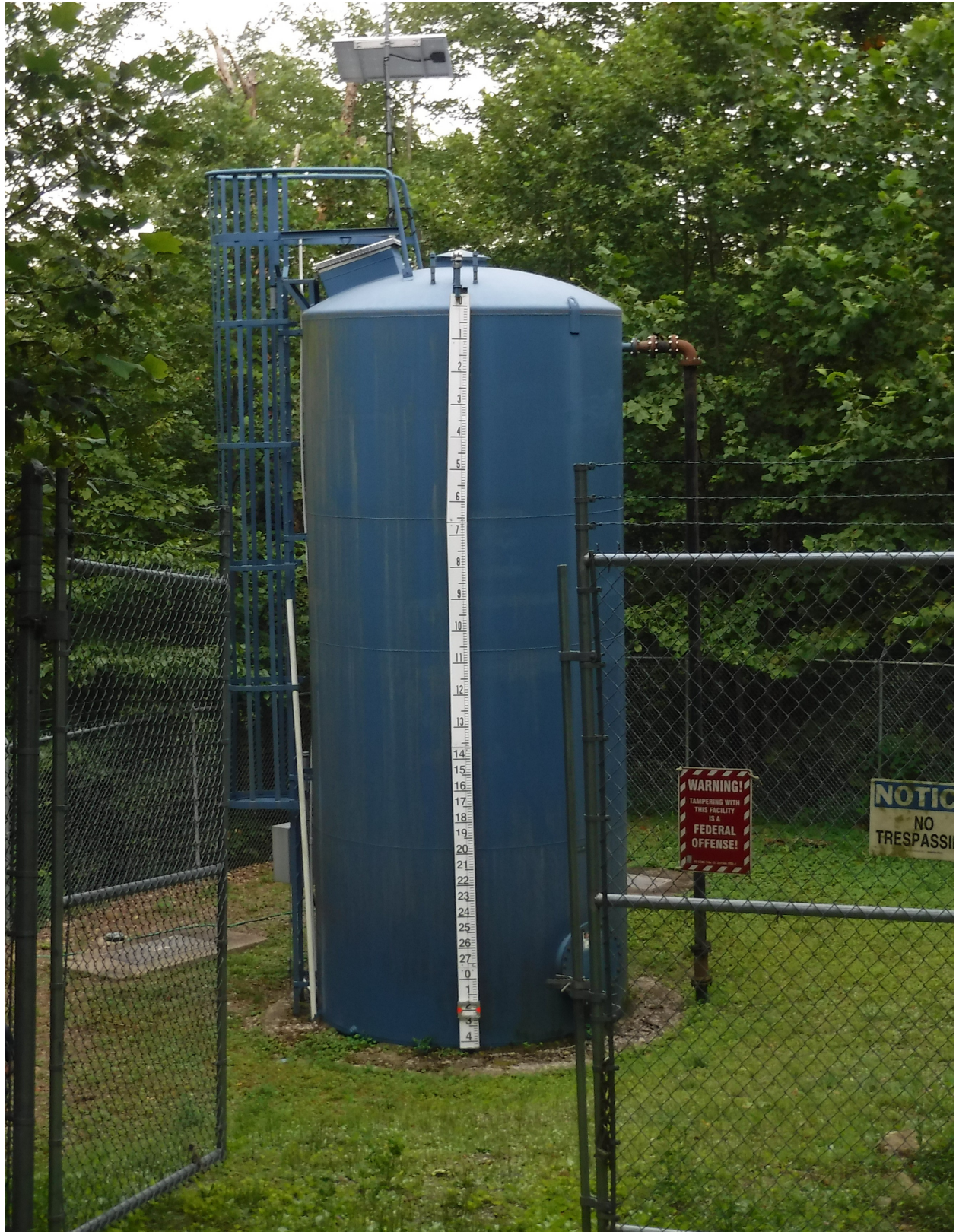
15,000 gallon standpipe located in Middlesboro, Kentucky and owned by Water Service Corporation of Kentucky.
