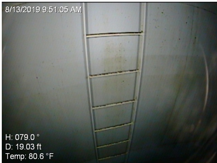
28) The wet interior ladder is in good condition. The ladder is not equipped with a fall prevention device.
