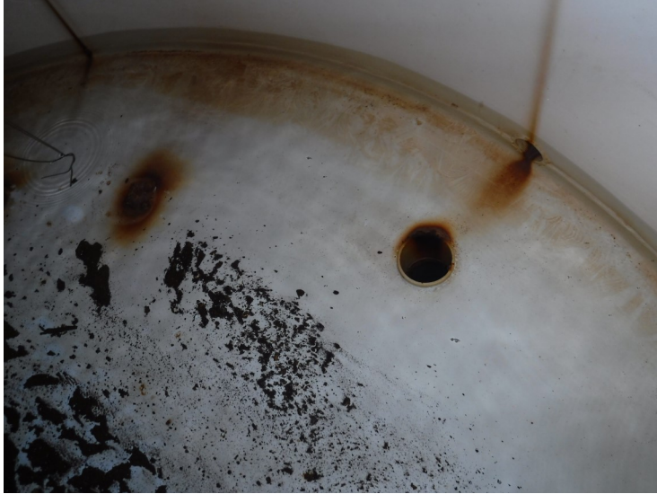
25) The draw pipe penetrates the floor and stubs just inside the wet interior.
