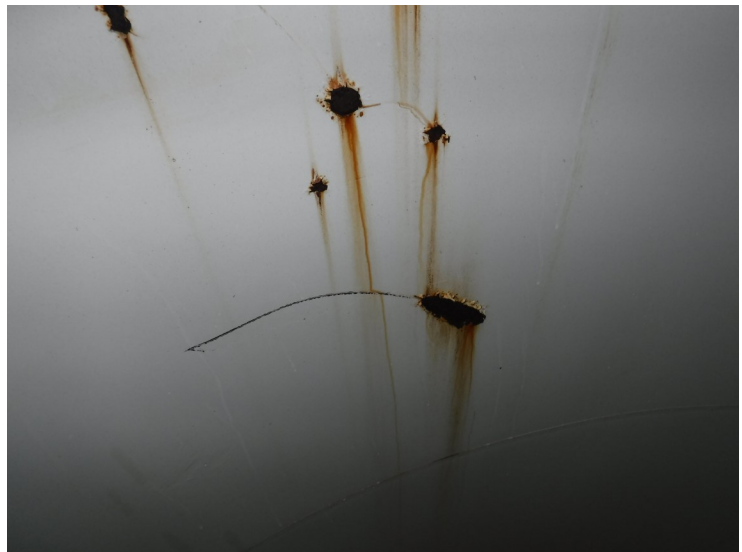
17) Spot coating failures on the sidewall.
