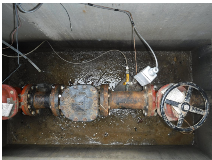
27) The pipe coating is in poor condition overall.
