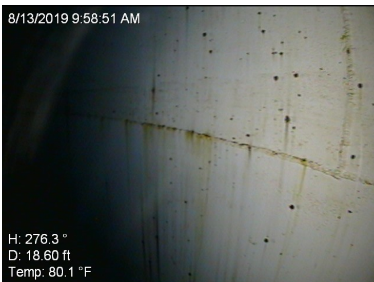
24) Spot coating failures on the sidewall.
