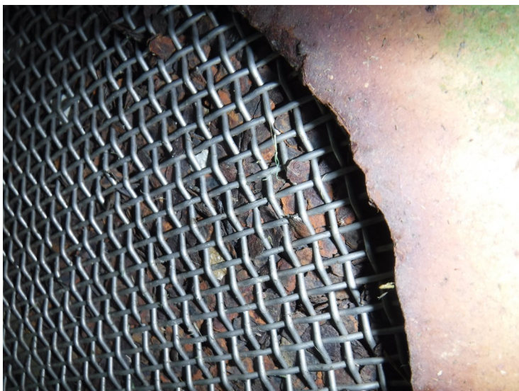
6) The overflow pipe discharge screen is partially plugged with debris.
