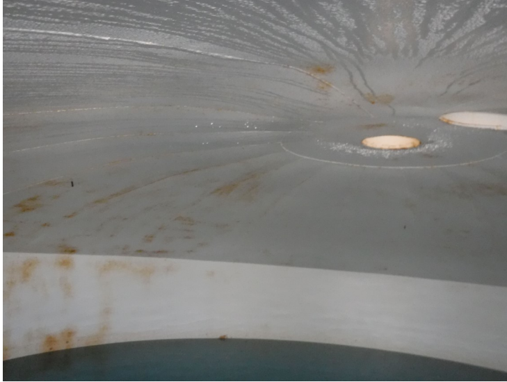
22) The wet interior roof coating is in fair condition overall with some rust bleedthrough.
