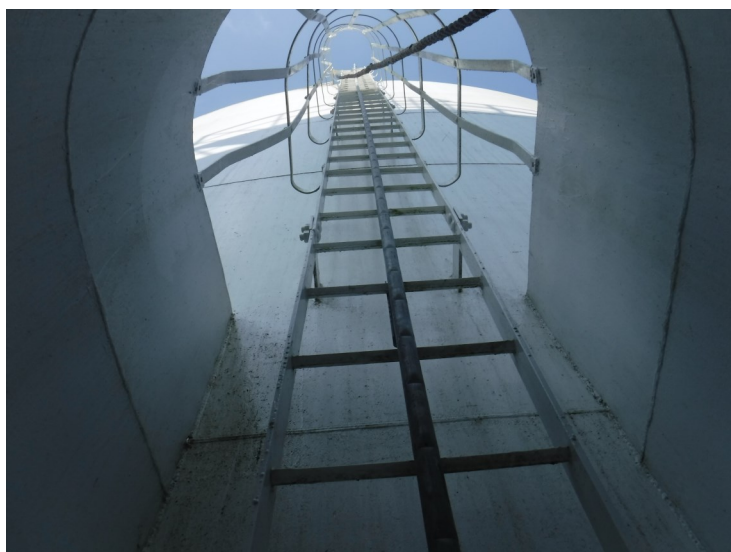
9) Sidewall ladder with rail-type fall prevention device.
