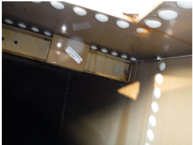
17) Liner deterioration at the roof supports and aerator supports.
