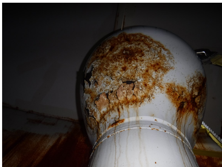
21) Coating failures on the overflow funnel.
