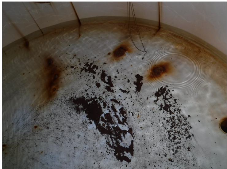
23) Spot coating failures on the floor.
