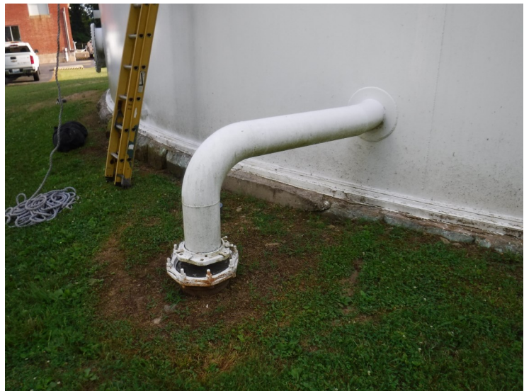
5) The overflow pipe discharges to a drain line that runs underground.
