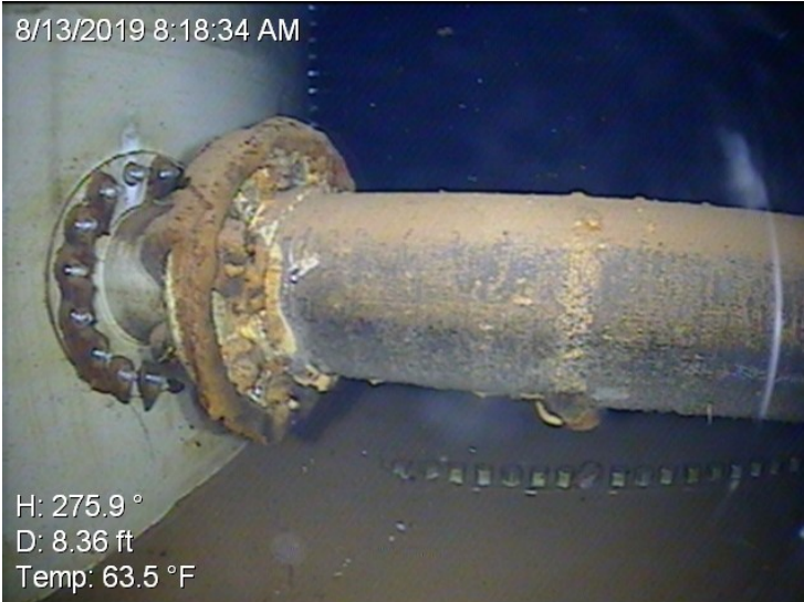
22) The fill pipe routes across the wet interior with some corrosion on the pipe and flanges.
