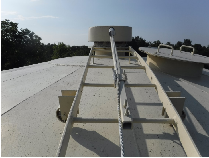
13) The roof ladder is in good condition and is equipped with a cable-type fall prevention device.
