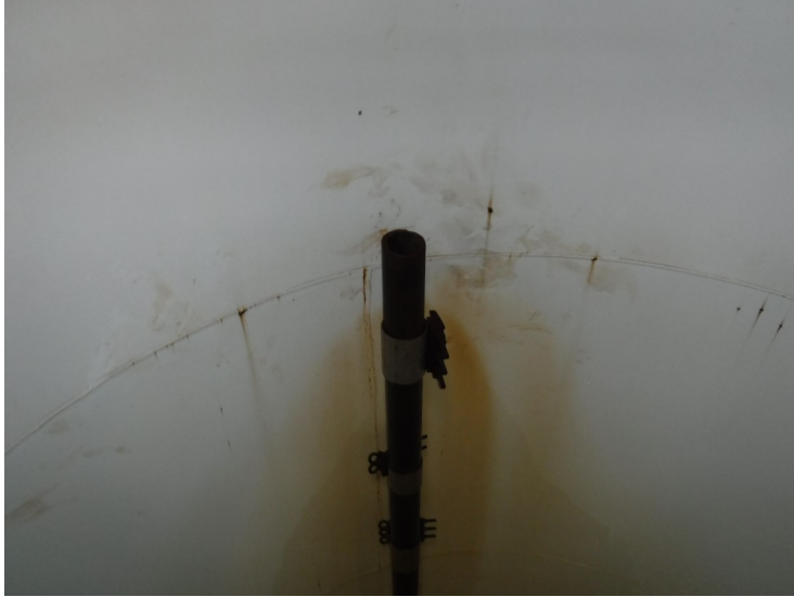
22) The fill pipe routes up the sidewall. The coating is in poor condition.
