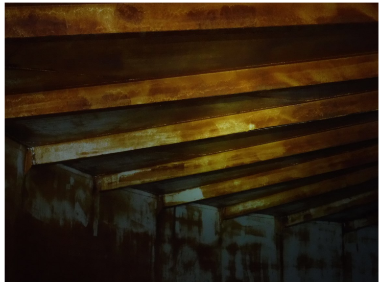
17) Extensive rust bleedthrough on the roof stiffener beams.
