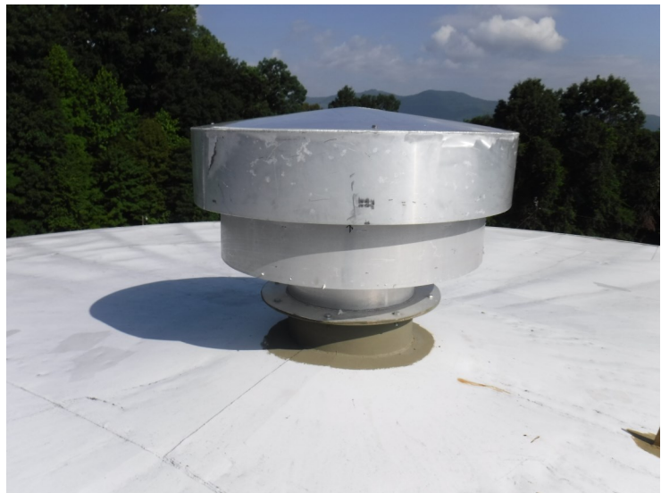
11) The frost free pressure vent is in good condition.
