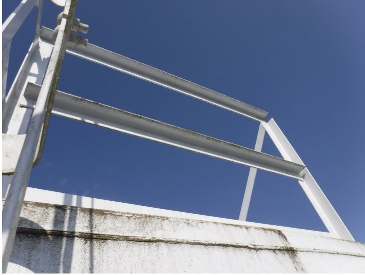
10) Roof handrail at the top of the ladder.
