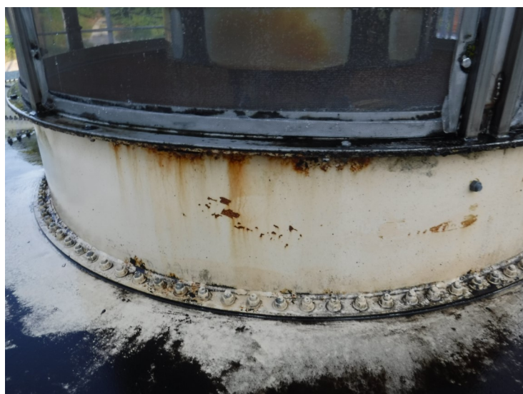
12) Spot lining deterioration on the aerator neck.
