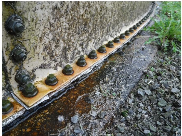
2) There are some sections of deteriorating felt pad filler.
