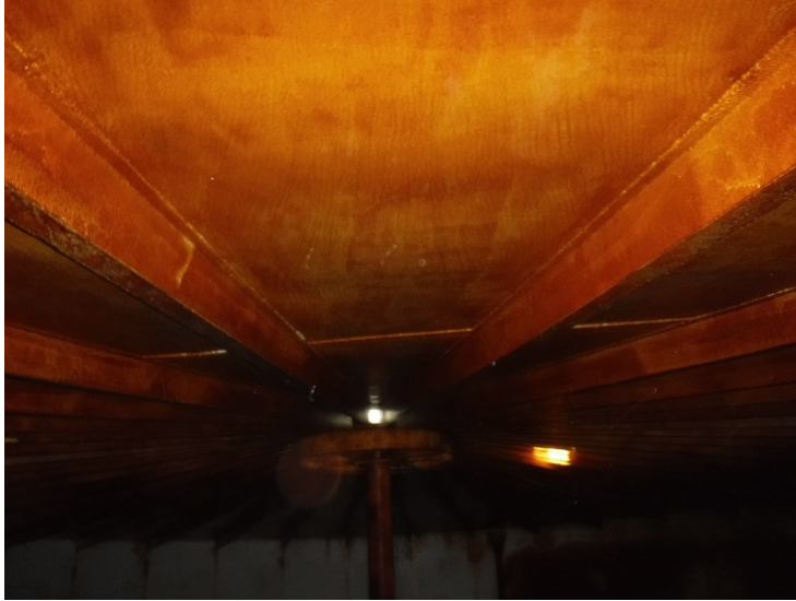
16) Extensive rust bleedthrough on the roof.
