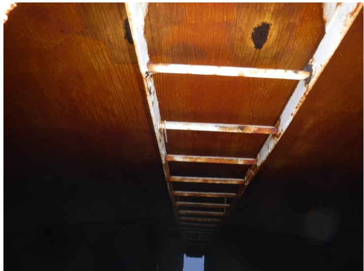
23) Wet interior ladder with rust bleedthrough and spot coating failures.
