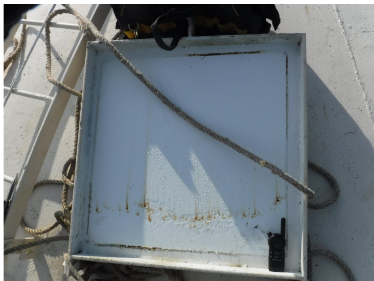
21) Spot coating failures on the inside of the hatch cover.
