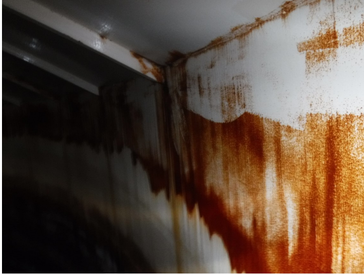
19) Rust bleedthrough along the upper sidewall.
