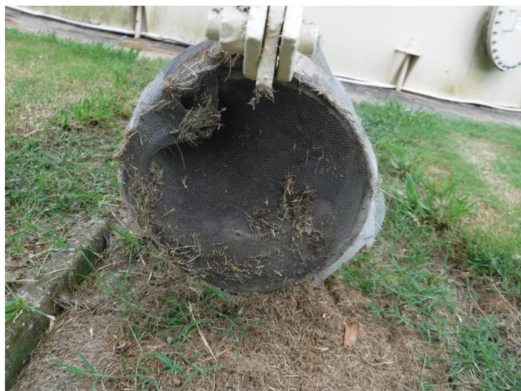
6) The overflow screen is in fair condition.
