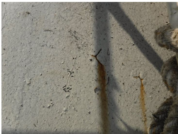
18) Spot coating failures with rust undercutting on the roof.
