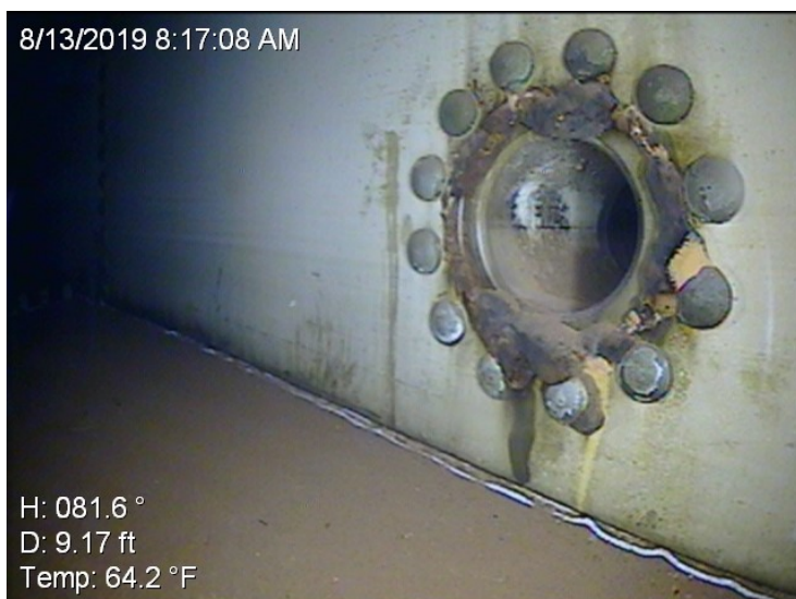
21) Drain penetration on the sidewall.
