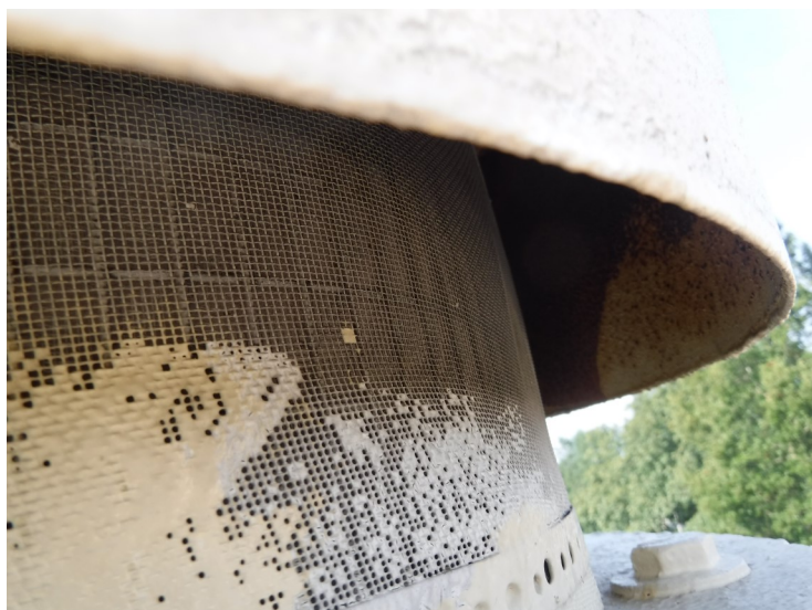
15) The roof vent screen is in fair condition and is partially coated.
