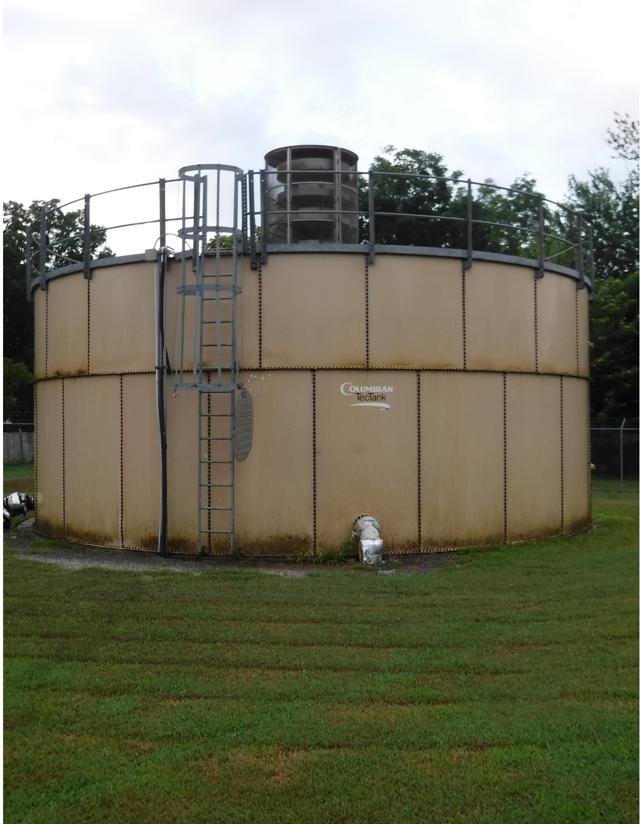
30,000 gallon reservoir located in Clinton, Kentucky and owned by Water Service Corporation of Kentucky.
