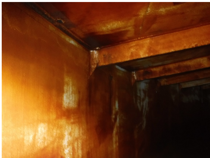
21) Extensive rust bleedthrough on the upper sidewall.
