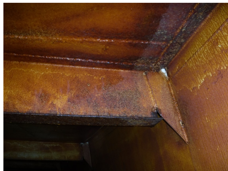
18) Edge corrosion on the roof stiffener beams.
