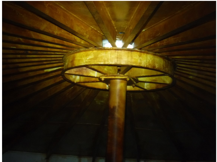
20) Rust bleedthrough on the center column.
