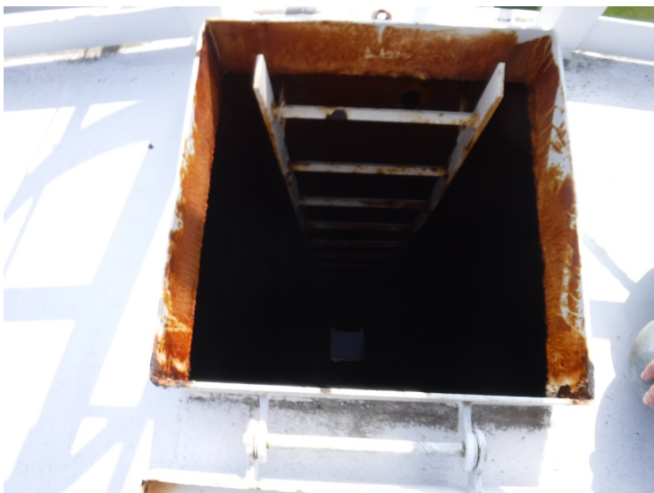
15) Rust bleedthrough on the wet interior hatch curb.
