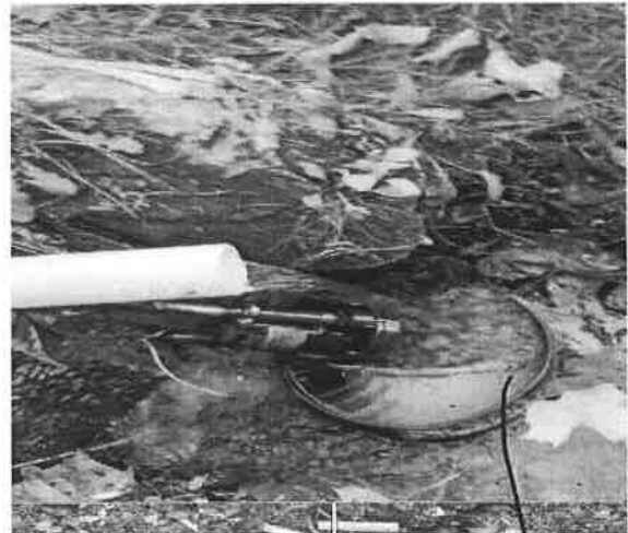
25GPM Leak customer catching and pumping to his house
