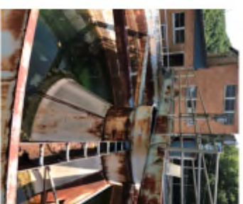
Failed Treatment Clarifier
