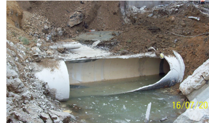
48" Water Main Break
