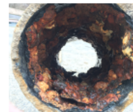
6" unlined cast iron pipe
