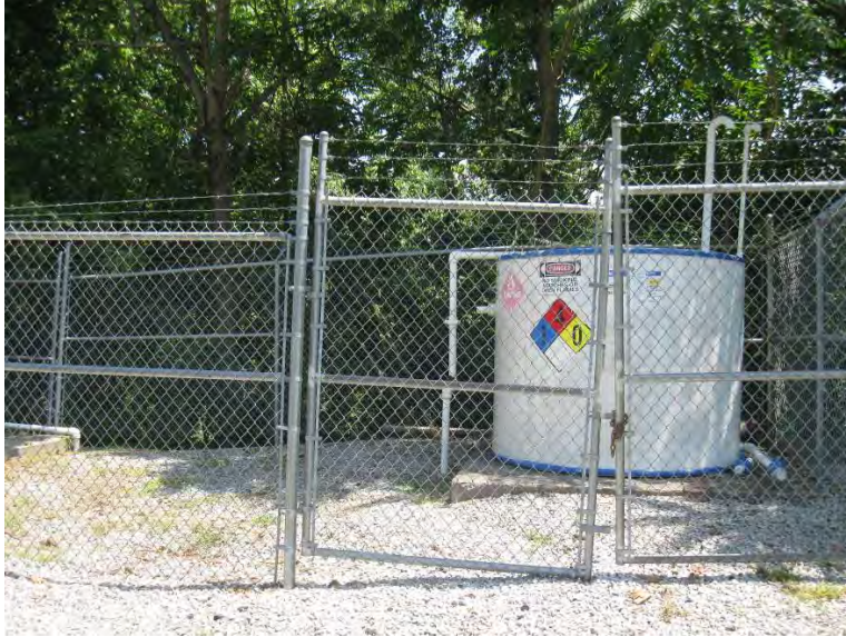
Photo No. 8 Right view of compressor station
