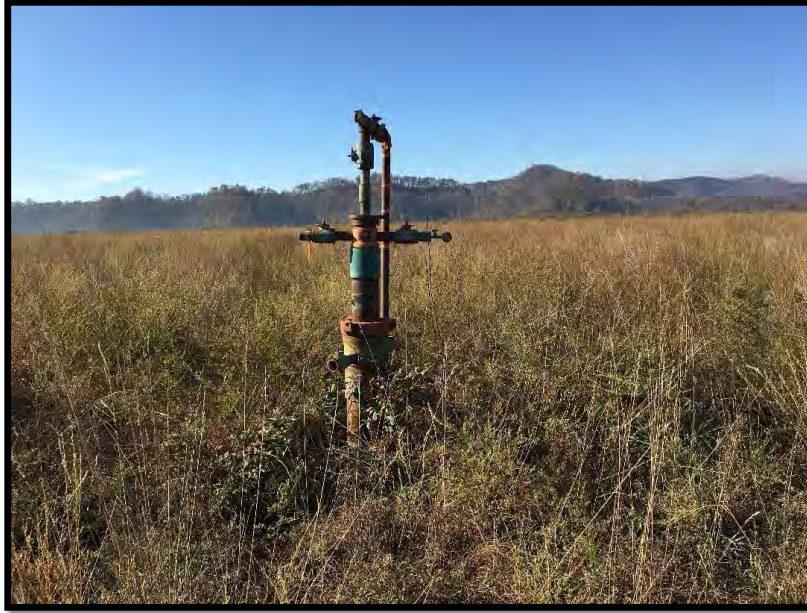
Photo #5 View of gas well transmission line.
