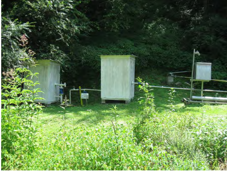
Photo No. 10 Gas well along sector #1 southern boundary
