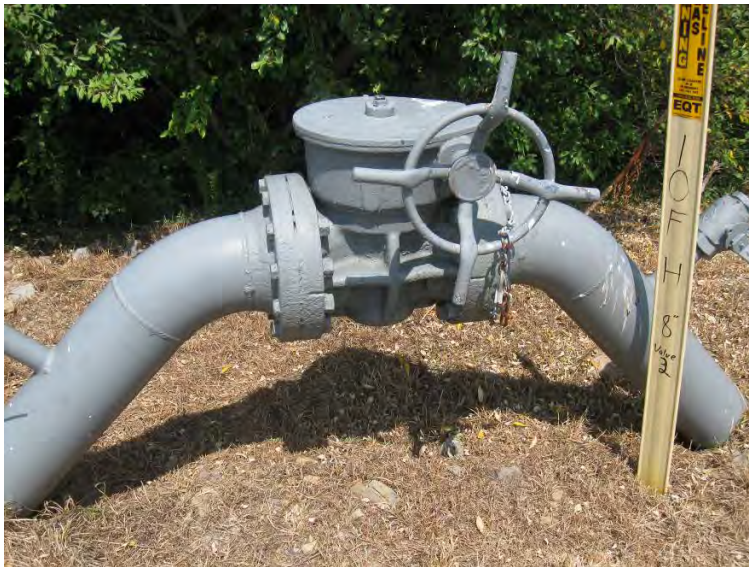
Photo No. 13 Exposed EQT gas line in sector #2
