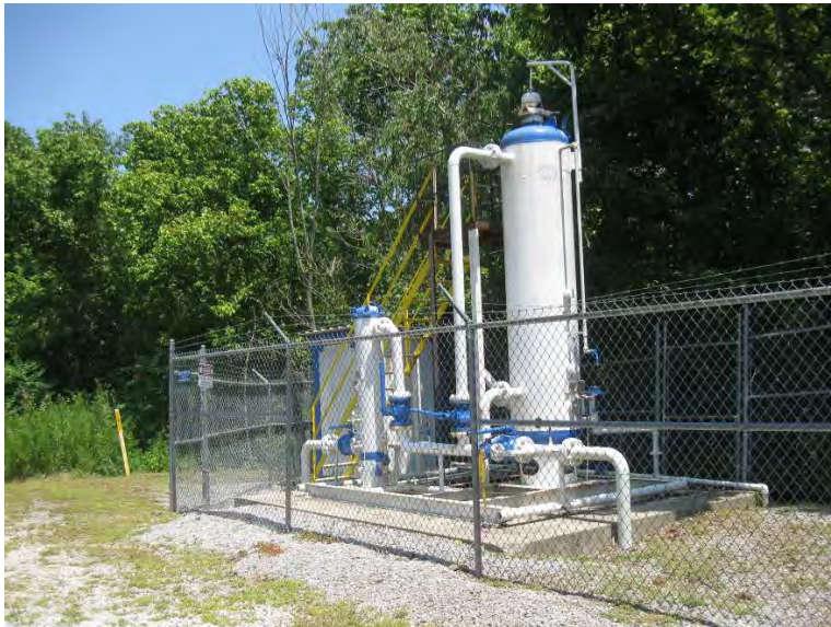
Photo No. 9 Left view of compressor station
