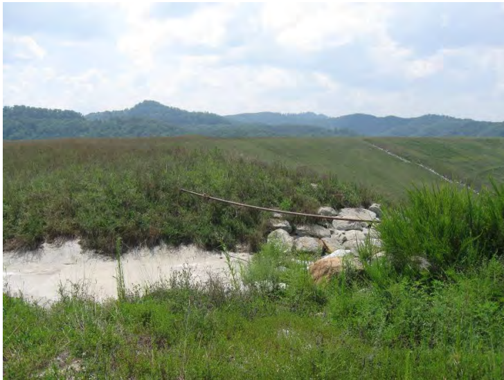
Photo No. 15 Exposed gas line in western portion of sector #2
