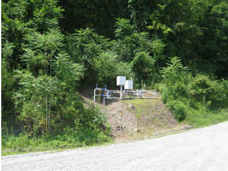
Photo No. 12 Exposed gas line adjacent to compressor station in sector #1
