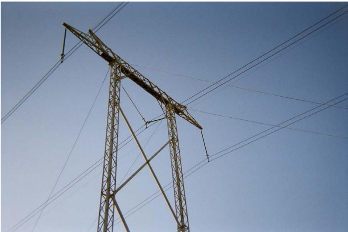
Figure 7.5 Corrugated Half-pipe Shielding Center Phase and Insulators from streamers. (Hérons can safely rebuild nests on top of the crossarm).
