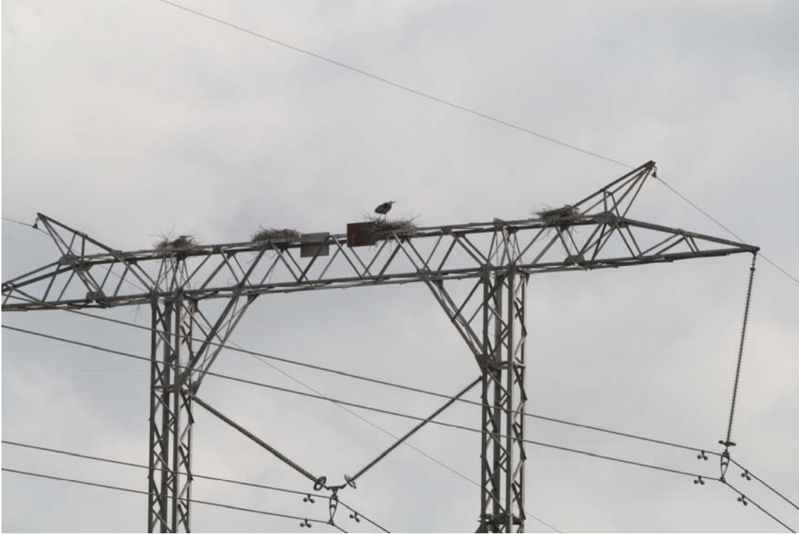
Figure 7.4 Heron nests on Transmission Tower (center phase and insulators contaminated)
