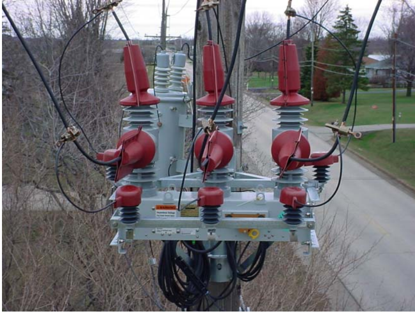
Figure 11.9 Transformer and Recloser Bushing Covers
