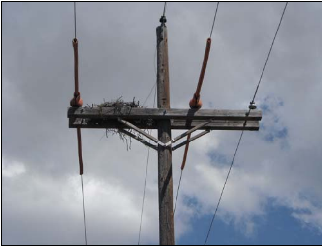
Figure 9.3 “Guts” covering the conductors where the hawks nest and perch.
