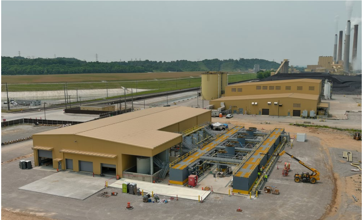
Ghent – ELG Water Treatment – June 2023
