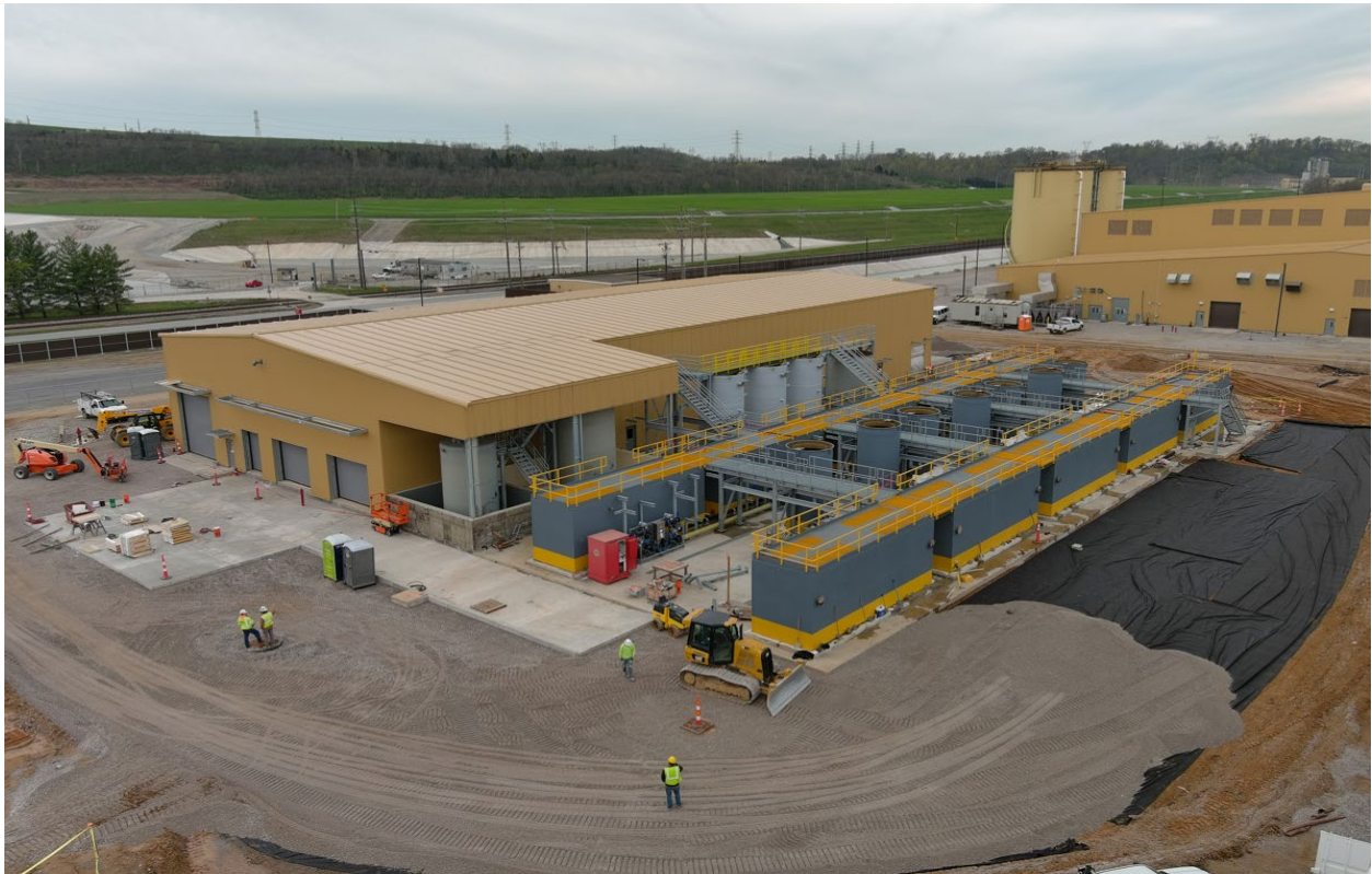
Ghent – ELG Water Treatment – April 2023
