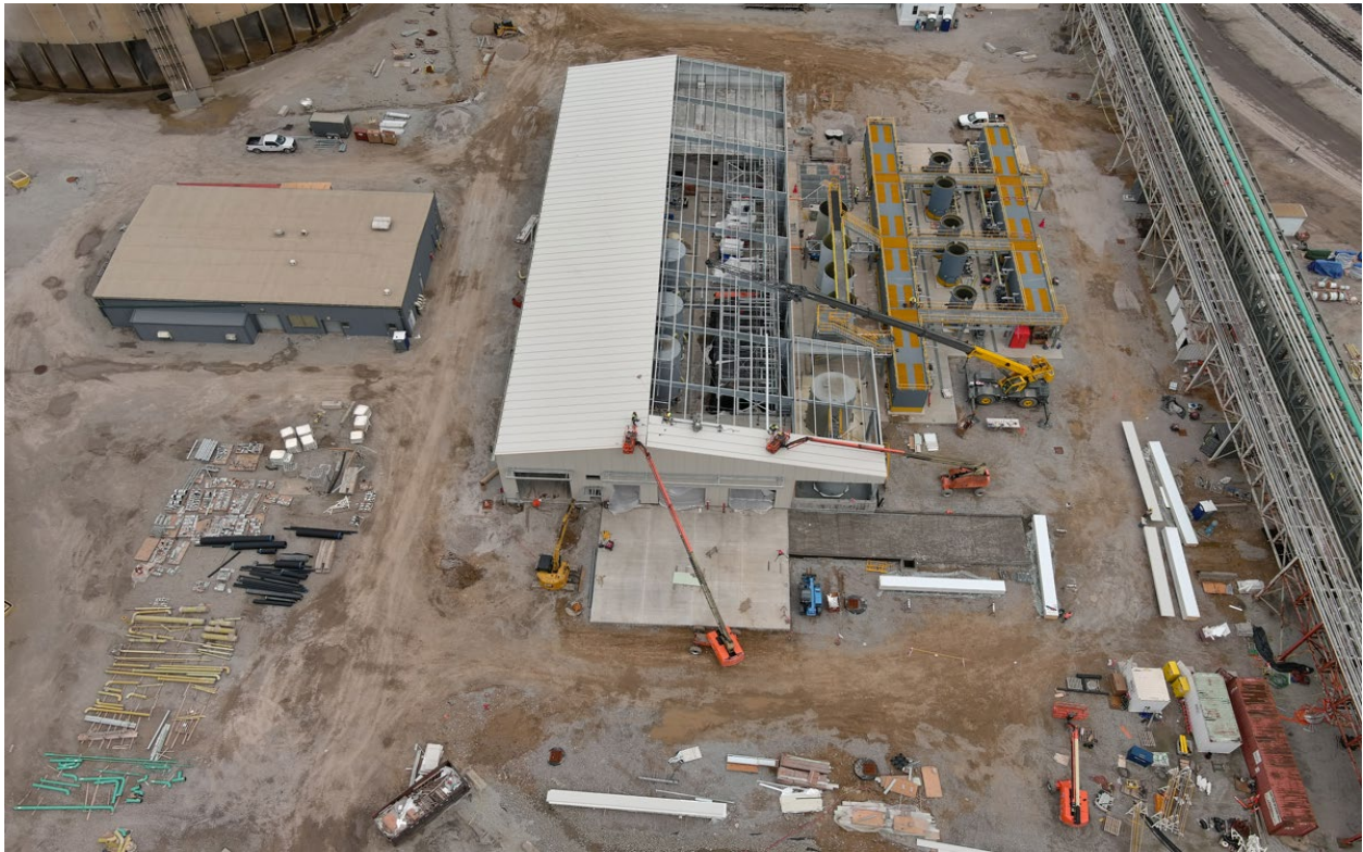
Mill Creek – ELG Water Treatment – April 2023
