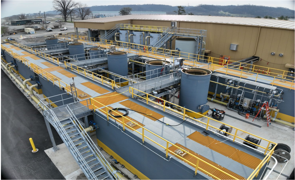
Ghent – ELG Water Treatment – March 2024
