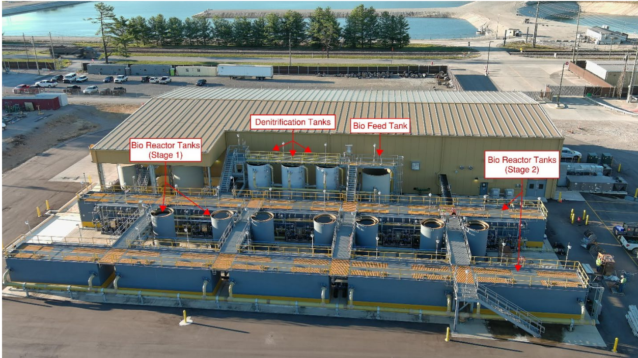
Ghent – ELG Water Treatment – July 2024
